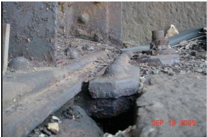
Figure 6.2.1r - Bearing worn into the bridge seat, needs to be shimmed and grouted
