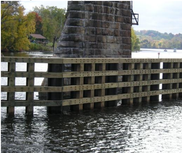
Figure 6.2.6.9i Newly installed fender system
