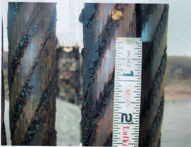
Figure 6.2.6.3p Counterweight ropes - severe crown wear
