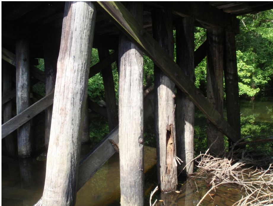
Figure 6.3.4a: Timber Bent with a pile – note decay damage
