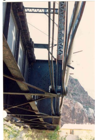
Figure 6.2.5d Bottom chord – loose eyebars (note bow in bars)
