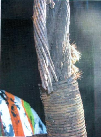
Figure 6.2.6.3o Counterweight ropes - broken strand
