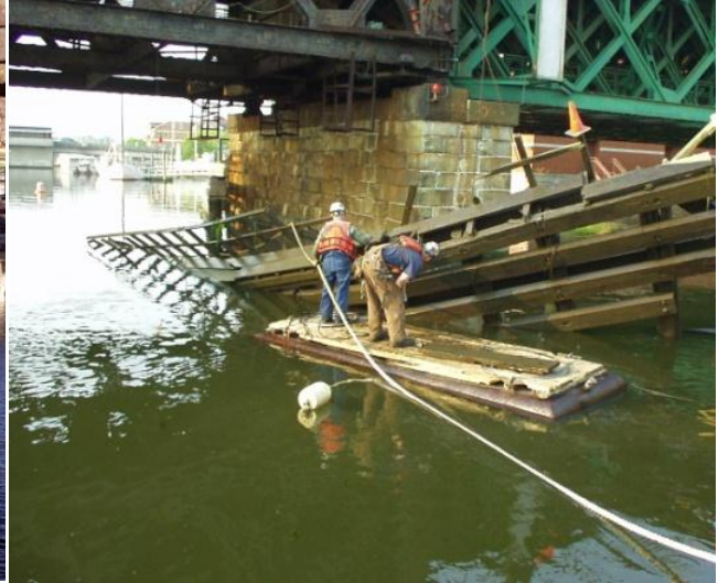
Figure 6.2.6.9h Failed fender system
