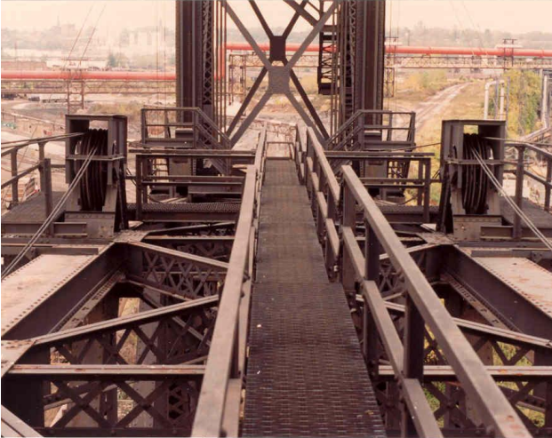
Figure 6.2.6.3r Operating ropes-idler wheels - excessive looseness in ropes
