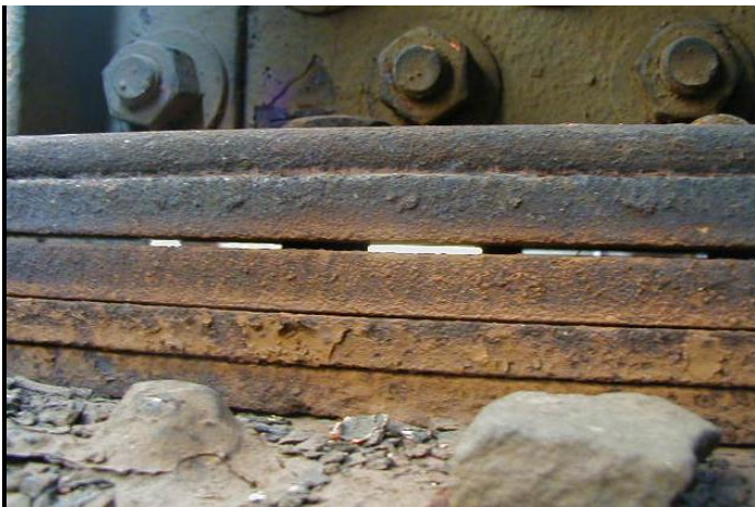
Figure 6.2.1q - Bearing with sole plate no longer in contact with masonry plate, needs to be shimmed and grouted
