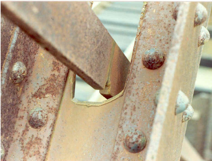
Figure 6.2.5e Pratt Truss – loose counter with section loss
