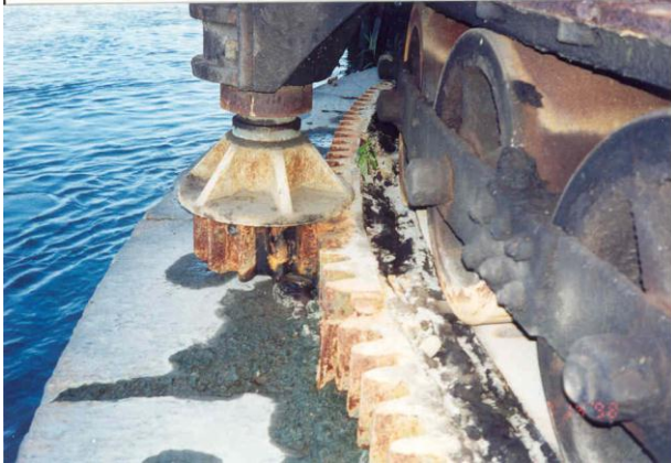
Figure 6.2.6.1j Rim support Rack/Drive Pinion - good alignment wheel protruding
