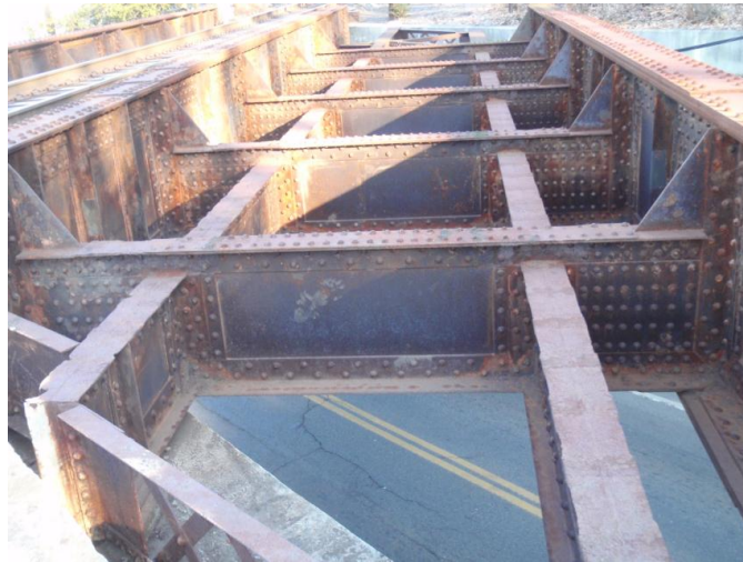
Figure 6.2.3.3.1a: Through Plate Girder with a Stringer Floorbeam System from the top, with the track removed
