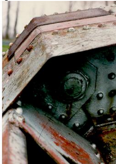
Figure 6.2.5c Joint U1 – hip joint patch plates over crack in bent plate joint movement
