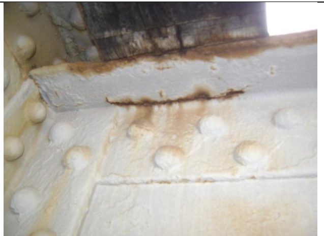
Figure 6.2.3.1d - Fatigue crack top flange angle
