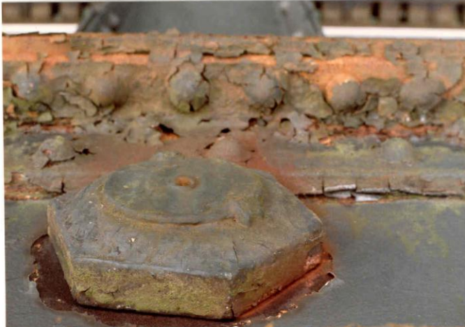
Figure 6.2.5g Slippage mark indicates amount of wear in joint
