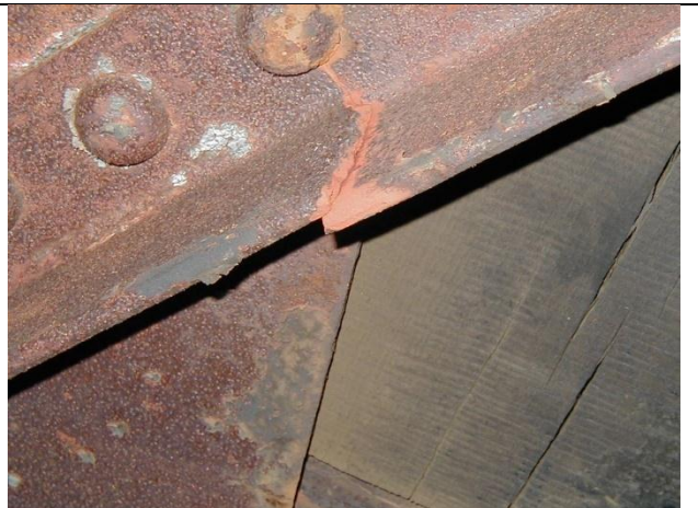
Figure 6.2.3.1f - Fatigue crack in a secondary member
