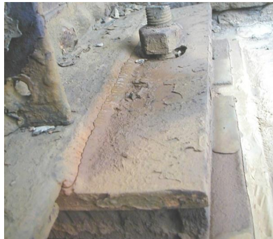
Figure 6.2.1v - Expansion bearing with cracked bottom flange to sole plate weld
