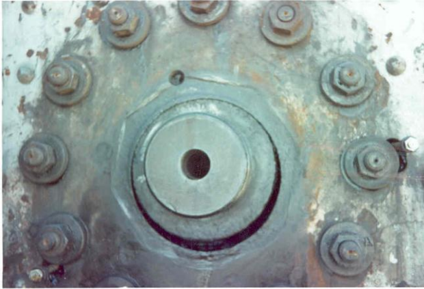
Figure 6.2.6.2m Strauss type bascule - counter weight trunnion joint, worn pin-gusset hole
