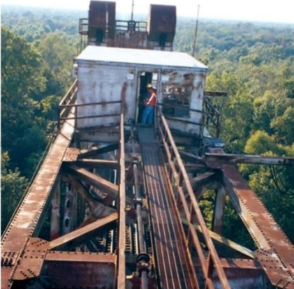
Figure 6.2.6.3s Span drive – bridge raised hood over sheaves (background) machine house and drive shaft (foreground)
