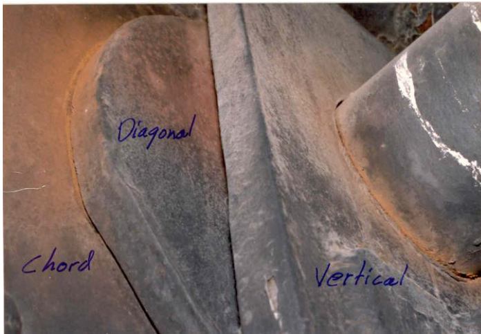
Figure 6.2.5i Interior of upper chord joint (note wear at pin and slippage between diagonal and chord)
