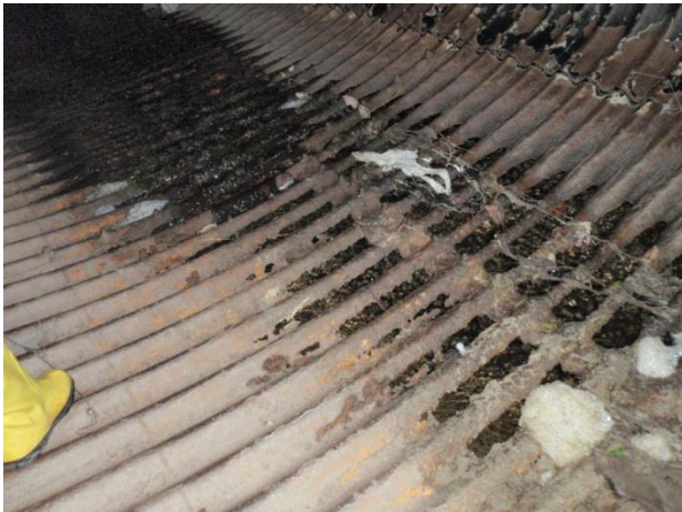
Figure 6.4g: Deteriorated bottom of a corrugated pipe culvert
