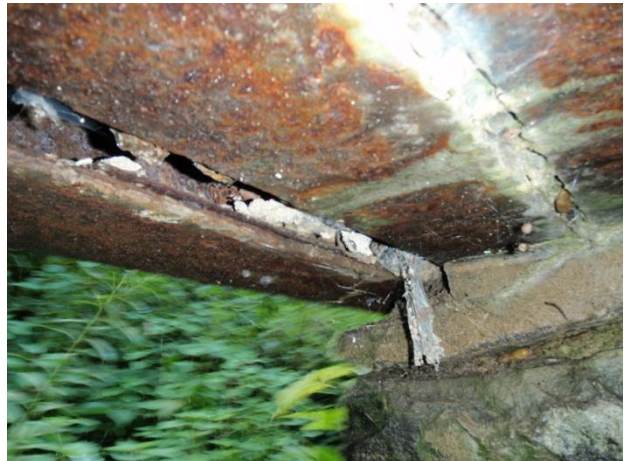
Figure 6.4h: Loss of concrete from slab above rail pipe culvert
