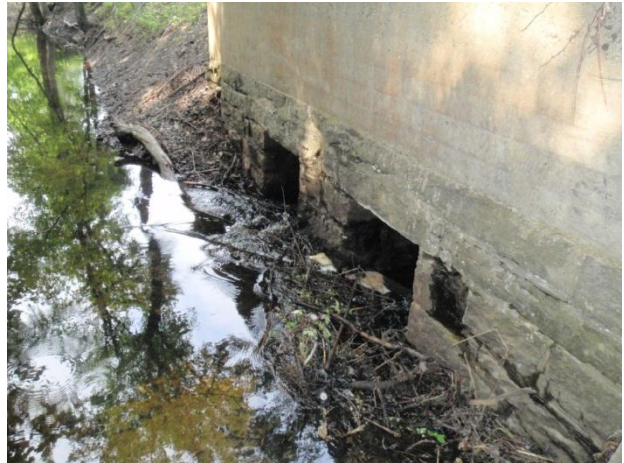
Figure 6.4f: Obstructed twin cell box culvert
