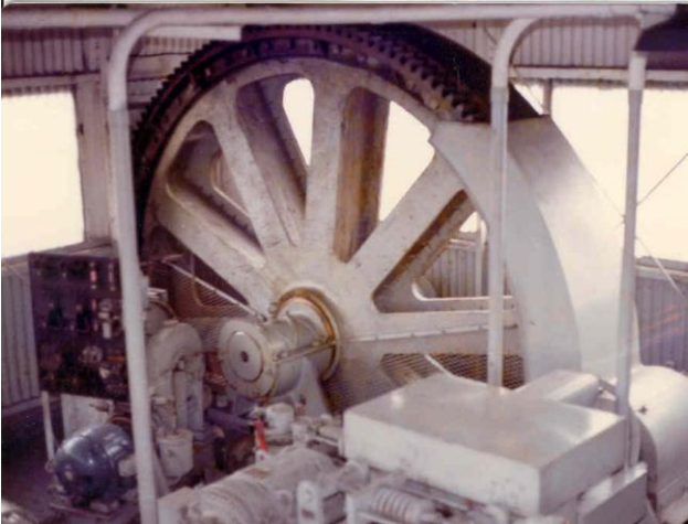
Figure 6.2.6.3h Sheave-bearing assembly tower drive trunnion bearings
