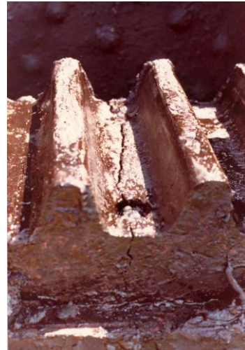
Figure 6.2.6.2l Rolling bascule - cracked rack section through bolt holes
