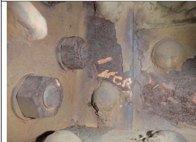
Figure 6.2.3.1c - Fatigue crack in a connect angle
