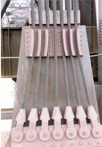
Figure 6.2.6.3m Counterweight ropes - cable splay at counterweight
