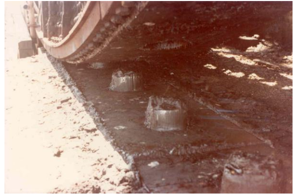
Figure 6.2.6.2h Rolling bascule - segment girder tread plate, worn pintles
