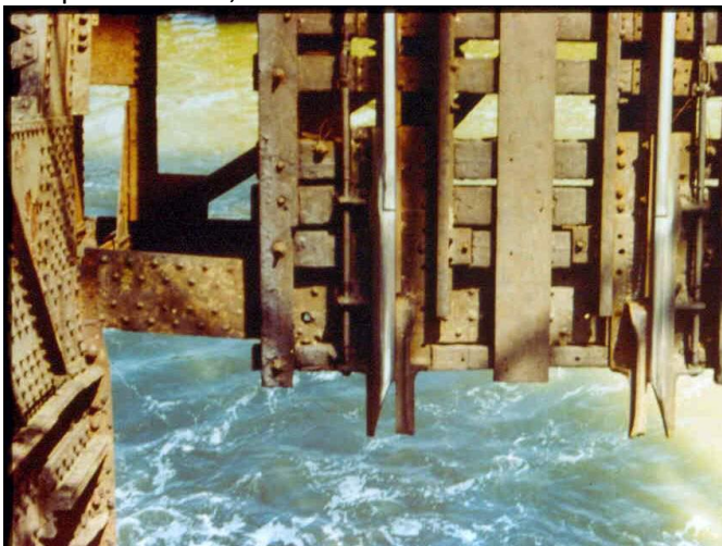
Figure 6.2.6.2q Bascule span – raised position Floorbeam – bowed from track load
