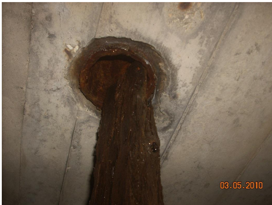
Figure 6.1.8a: A deck wheephole blocked by a piece of timber
