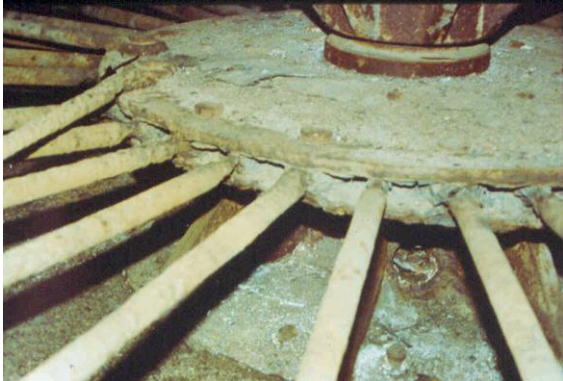
Figure 6.2.6.1h Rim support spider rod - section loss at center connection plate
