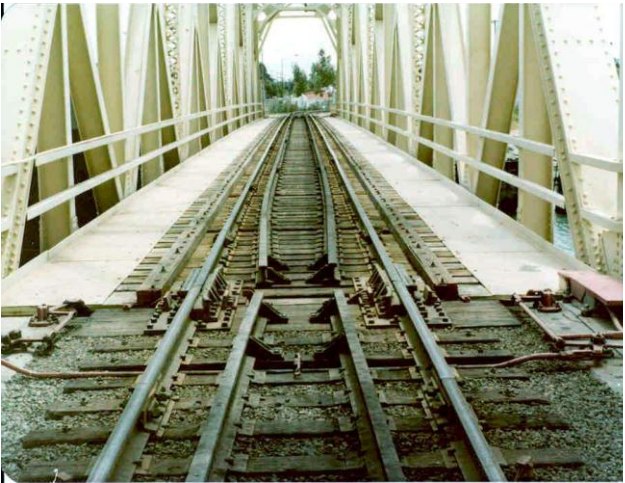
Figure 6.2.6.3x Two-piece miter rail and signal equipment
