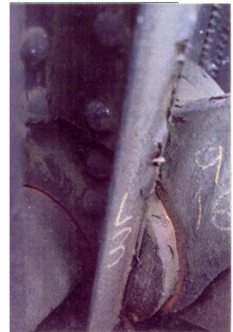
Figure 6.2.5j Lower pin joint slippage marks indicate wear in components
