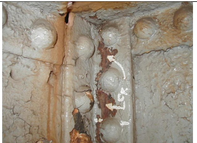
Figure 6.2.3.1b - Fatigue crack in a connection angle
