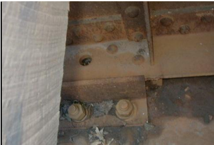
Figure 6.2.1u - Expansion bearing with deteriorated anchor bolt, replaced with steel angle keeper system
