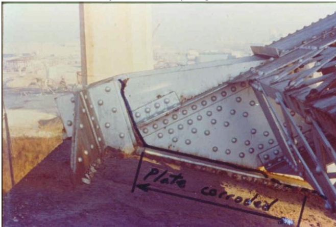
Figure 6.2.6.2o Strauss type bascule - counter weight hip connection, crack due to interface corrosion
