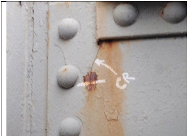
Figure 6.2.3.1a - Fatigue crack in a diaphragm web
