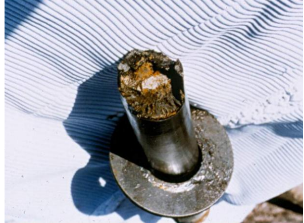
Figure 6.2.6.2n Strauss type bascule - broken retain bolt, common with joint wear
