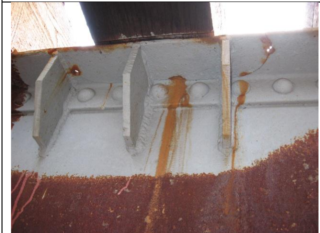
Figure 6.2.3.1e - Fatigue crack top flange angle with stop holes drilled and repair stiffeners installed
