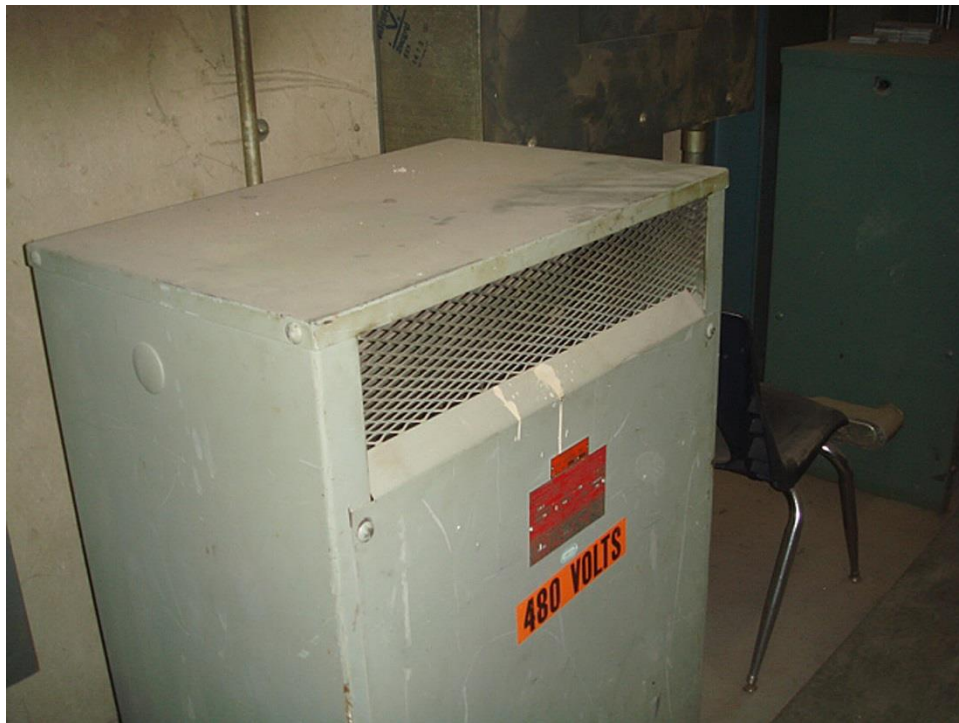
Main Electric Service
