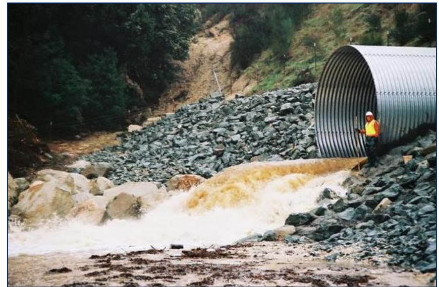
Image of rock energy dissipater. California Department of Transportation. Office of Hydraulics and Stormwater Design. Retrieved from http://www.dot.ca.gov/design/hsd/index.html
