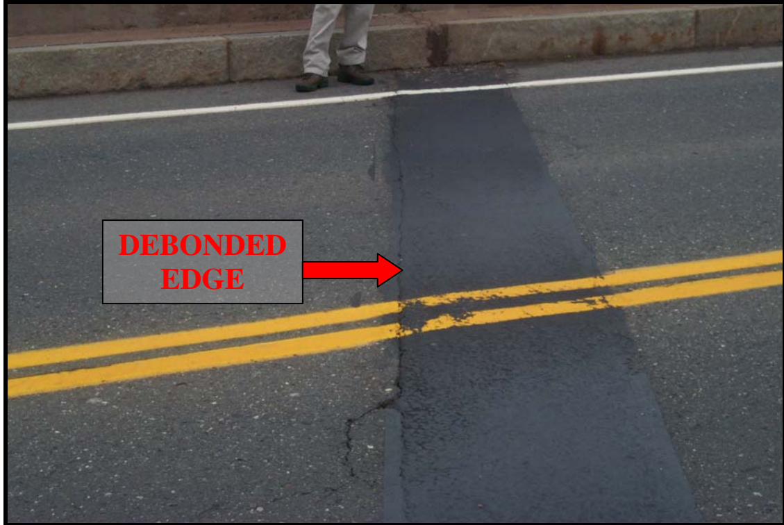
Picture #9: Debonding on bridge #03163 RTE. 160 over I-91 Rocky Hill, CT
