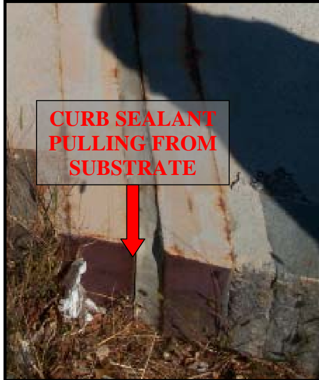
Picture #4: Curb Sealant Issues on bridge #W06053 North Street Over I-195, Wareham, MA
