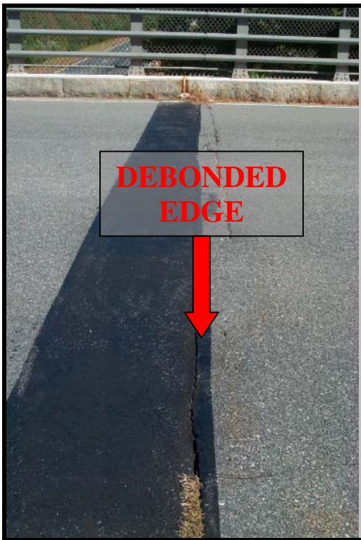
Picture #10: Debonding on bridge # M09009 Route 28 over I-195 Mattapoisett, MA
