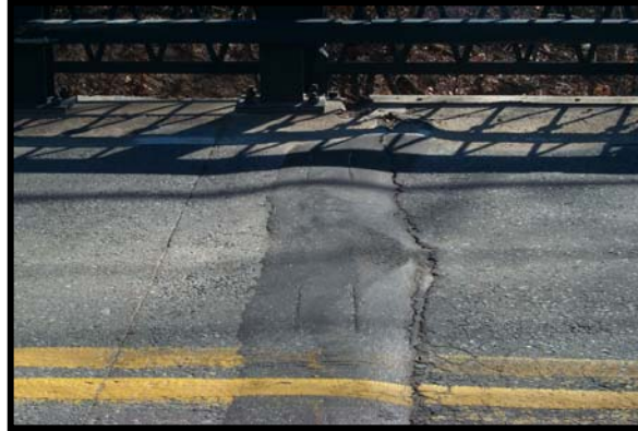
Picture #32: No Curb on Bridge #164 School Street over Blackstone River Lincoln Cumberland, RI
