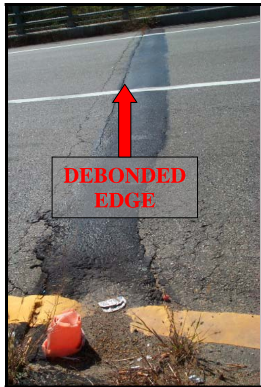
Picture #11: Debonding on bridge # W06053 North Street over I-195 Wareham, MA
