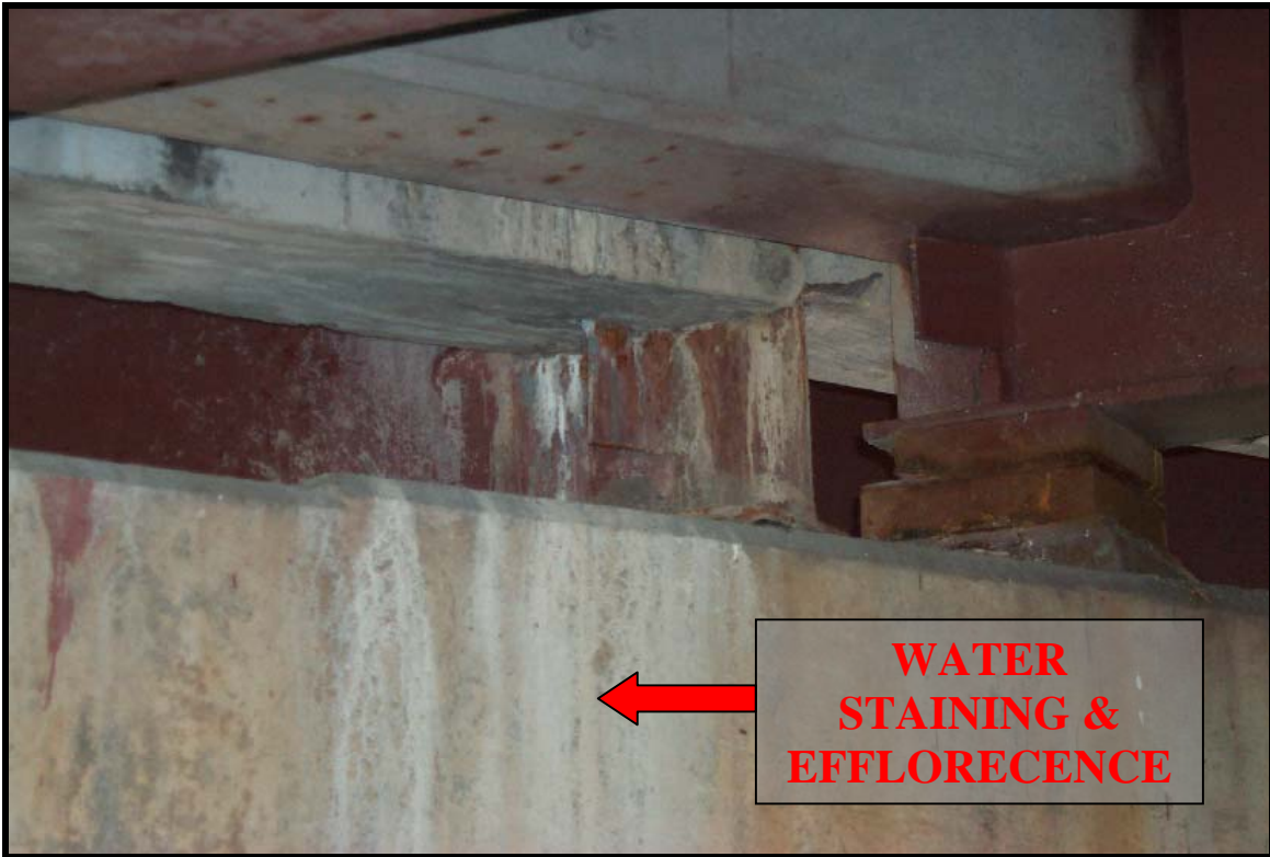
Picture #14: Water staining on bridge#N06013 Route 140 over Braley Road New Bedford, MA
