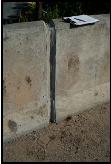
Picture #28: Parapet Detail on Bridge#W30025 I-195 West over Sanford Road Westport, MA
