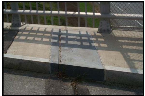
Picture #31: Custom Curb Detail on Bridge#102/120 Old Route 16 over Branch River Milton, NH
