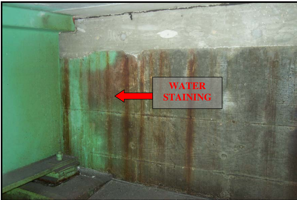
Picture #15: Water staining on bridge#102/120 Old Route 16 over Branch River Milton, NH
