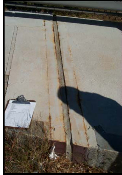
Picture #29: Standard Curb Detail on Bridge #W06053 North Street over I-195 Wareham, MA
