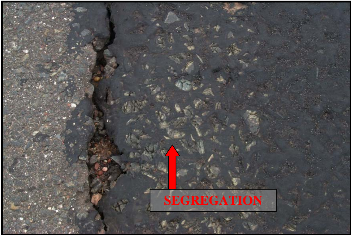
Picture #22: Segregation on bridge #03313 I-84 TR Over 815 New Britain, CT
