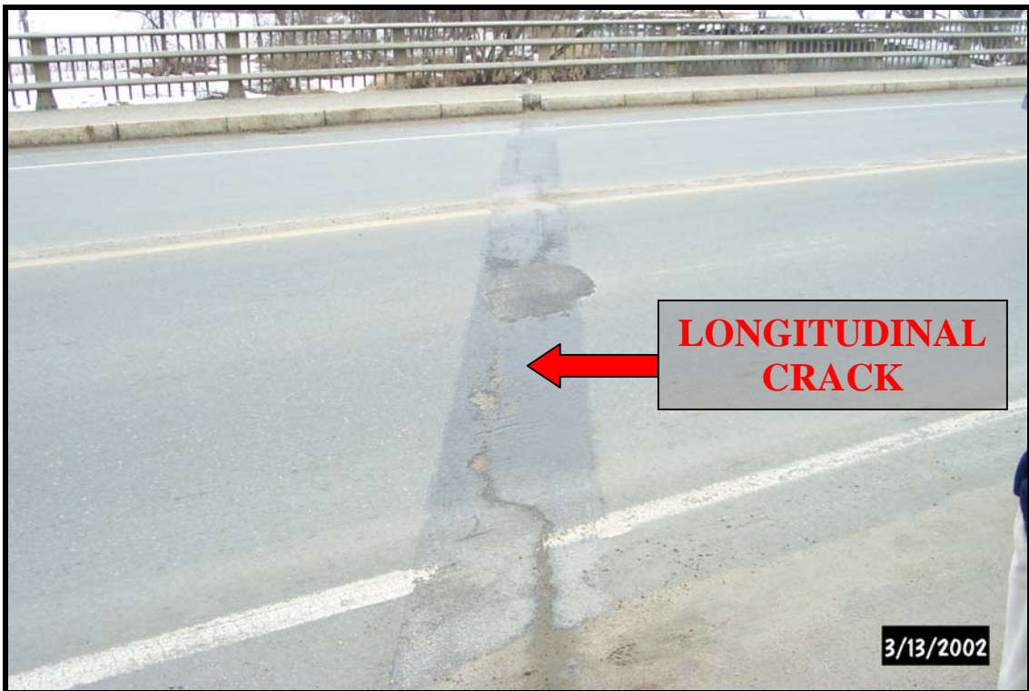
Picture #6: Cracking on bridge#144 US 5/Passumpsic River Joint 2 Lyndon, VT
