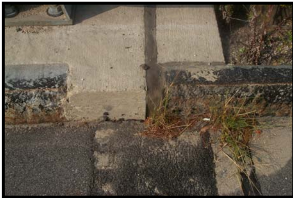
Picture #30: Sliding Plate Detail on Bridge#123/173 NH Route 27 over NH Route 101 Hampton, NH
