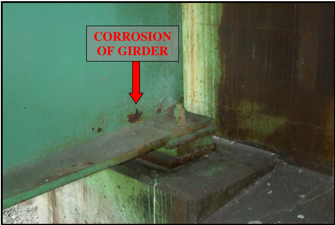
Picture #16: Girder corrosion on bridge #102/120 Old Route 16 over Branch River Milton, NH
