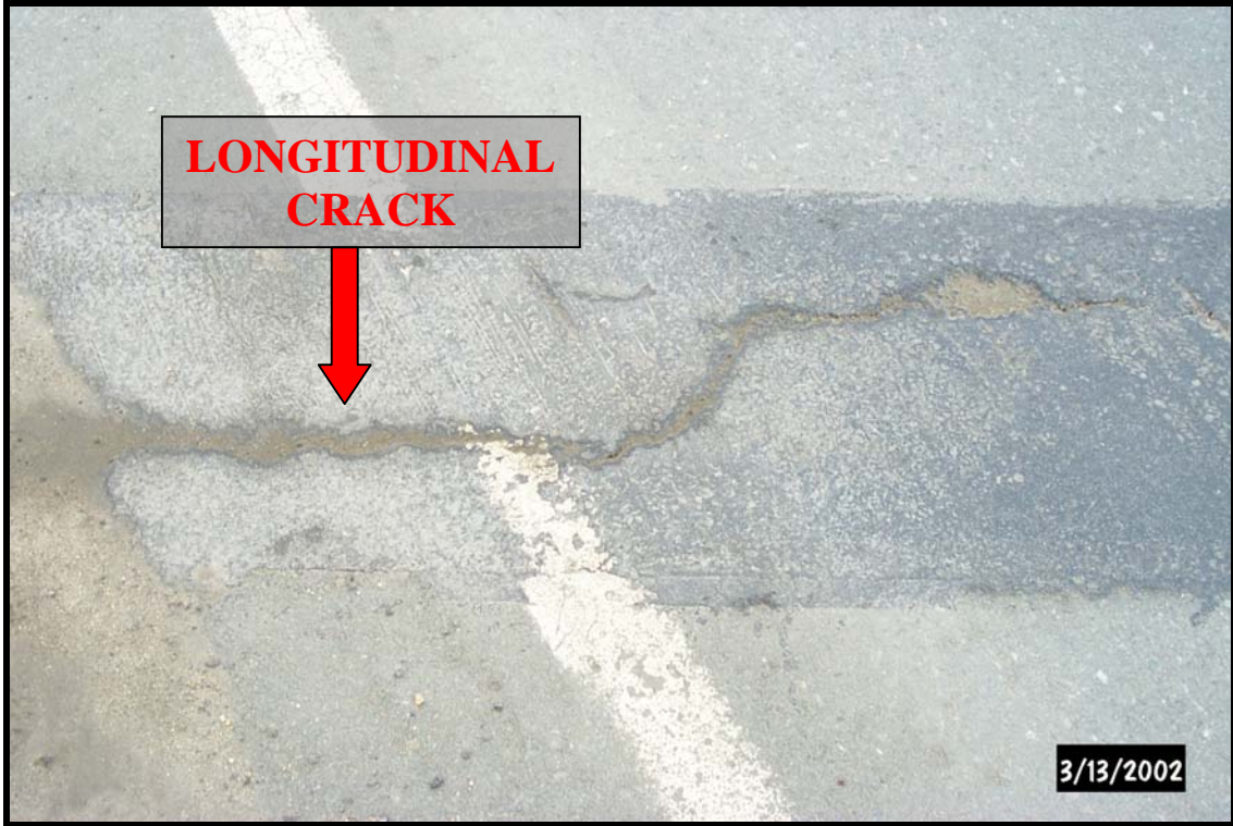
Picture #5: Cracking on bridge#144 US 5/Passumpsic River Joint 2 Lyndon, VT
