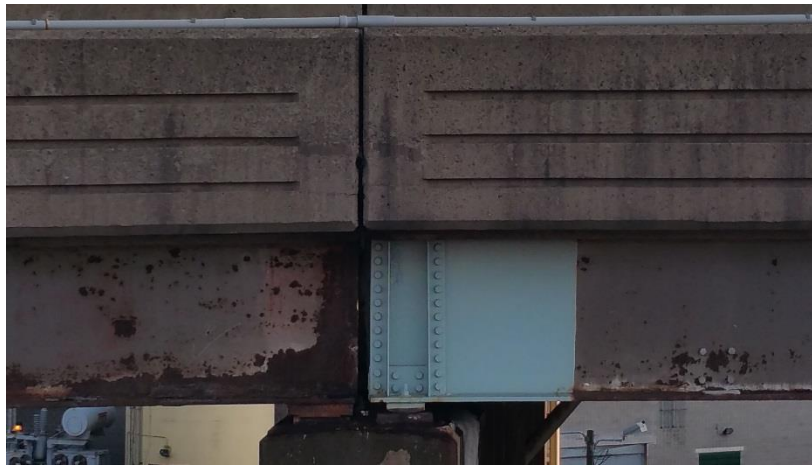
Figure 1.2: Corrosion damage and conventional repair method
