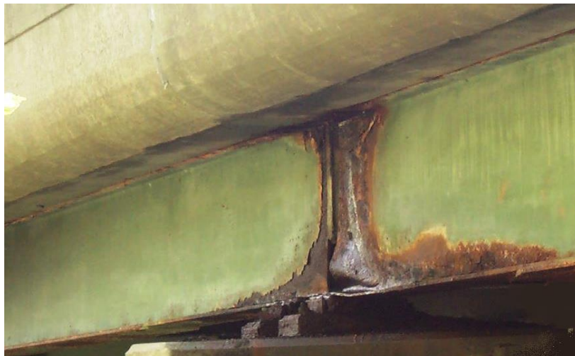
Figure 1.1: Typical corrosion damage of girder ends beneath the expansion joint
