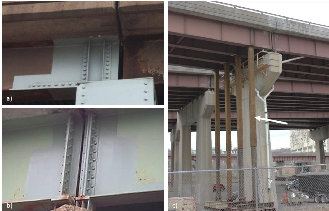
Figure 1.3: Conventional Repair Method for corroded girder ends including jacking of the superstructure during construction
