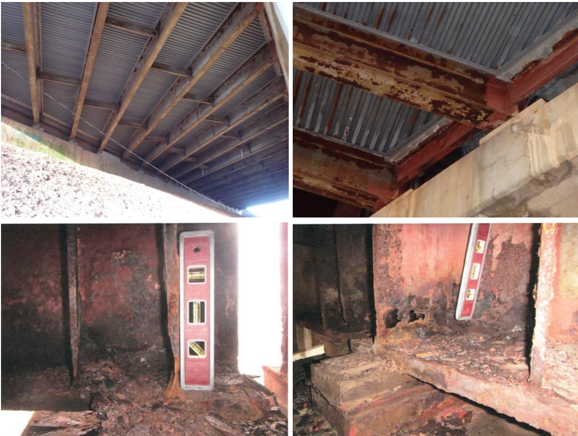
Figure 5.2: Severe corrosion damage of girder ends
