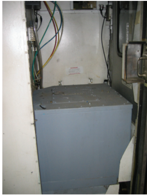
Typical Metro-North re-circulating system holding tank
