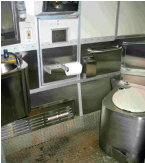
Bombardier Car (Shoreline East) - ADA lavatory overview
