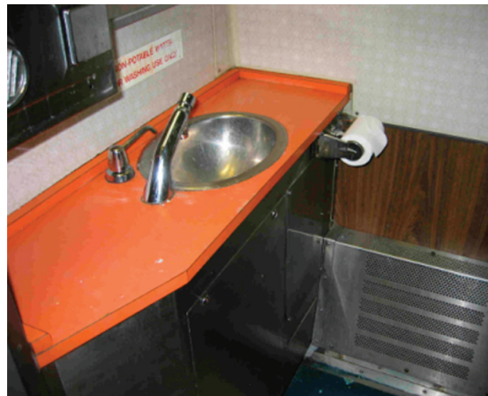
M-4 re-circulating system sink and counter
