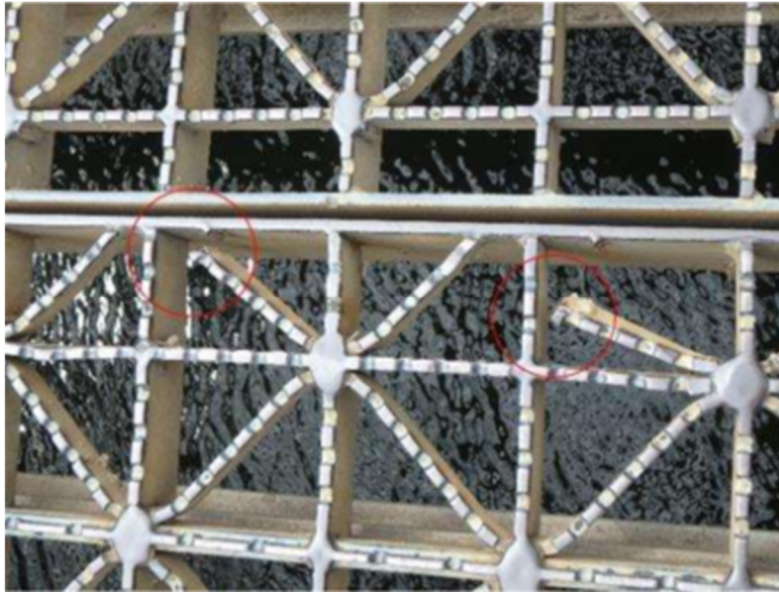
Steel Grid Deck has broken Diagonal Bars Between Floorbeams 2 & 3 and Stringers 3 & 4
