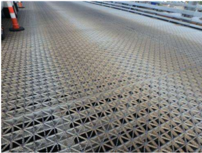
Steel Grid Deck with Areas of Peeling Galvanized Coating
