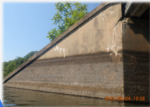
Southeast Wingwall, note cracking and efflorescence (mineral deposits)
