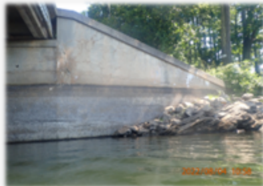
Northeast Wingwall, note cracking, efflorescence (mineral deposits)
