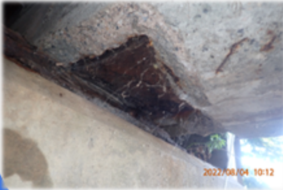
Concrete encasement broken off at end of beam, negligible section loss
