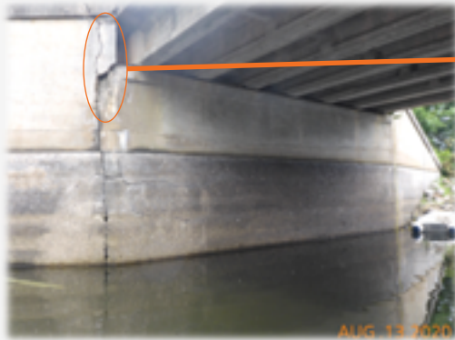
Abutment 2 with cracking and spalling (crumbling off)
