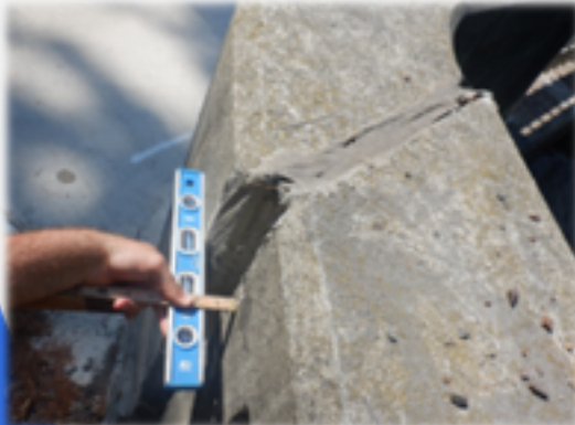
Northwest wingwall barrier is misaligned >1-1/2"
