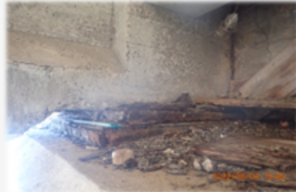
Steel Bearings with heavy laminated and pack rust
