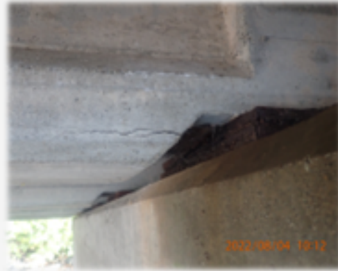
Concrete encasement cracking at end of beam
