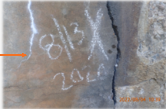
Crack up to 1.25" displacement
