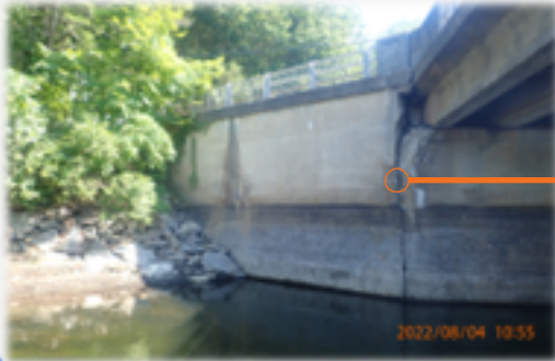
Northwest Wingwall, note cracking, efflorescence (mineral deposits) and spall (crumbling concrete)
