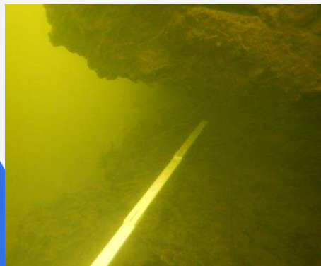
Void at Pier 7
