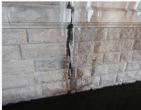
Longitudinal Joint at Pier 3
