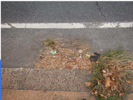
Clogged Deck Drains
