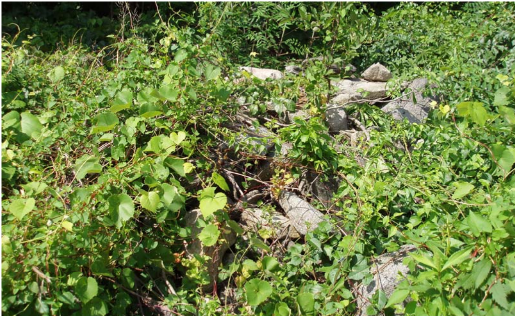
Figure No. 17: Southwest view of remains of ca. 1880 Louis J. Van Hoesen Hotel, overgrown with scrub growth after having been recently burnt down and razed.
