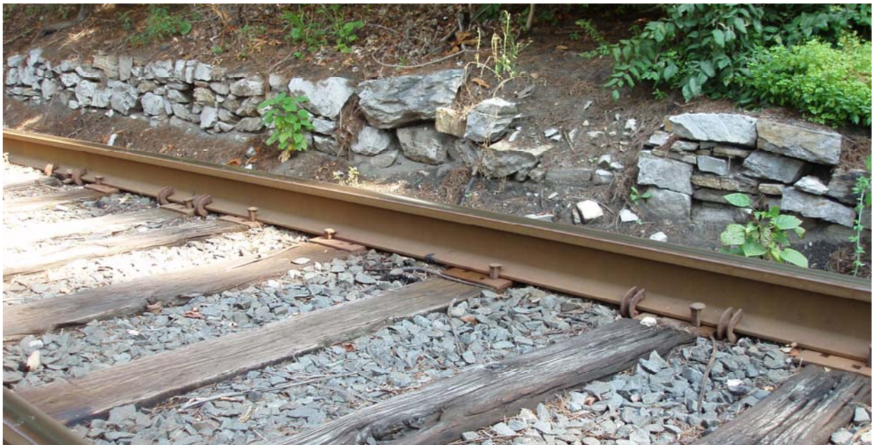
Figure No. 21: Northeast view of retaining wall on east side of tracks in New Milford, constructed from roughly coursed marble. RR feature #9.
