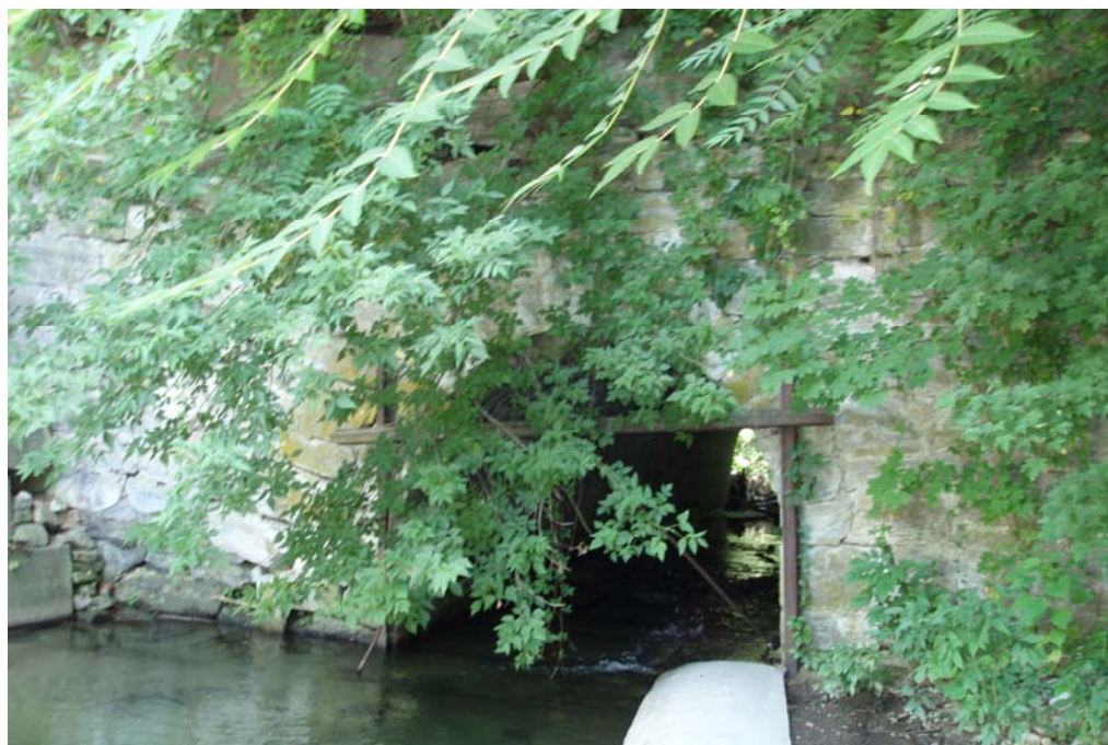
Figure No. 19: East view of the arched tunnel under the railroad line near West Street in New Milford at the Great Brook crossing.
