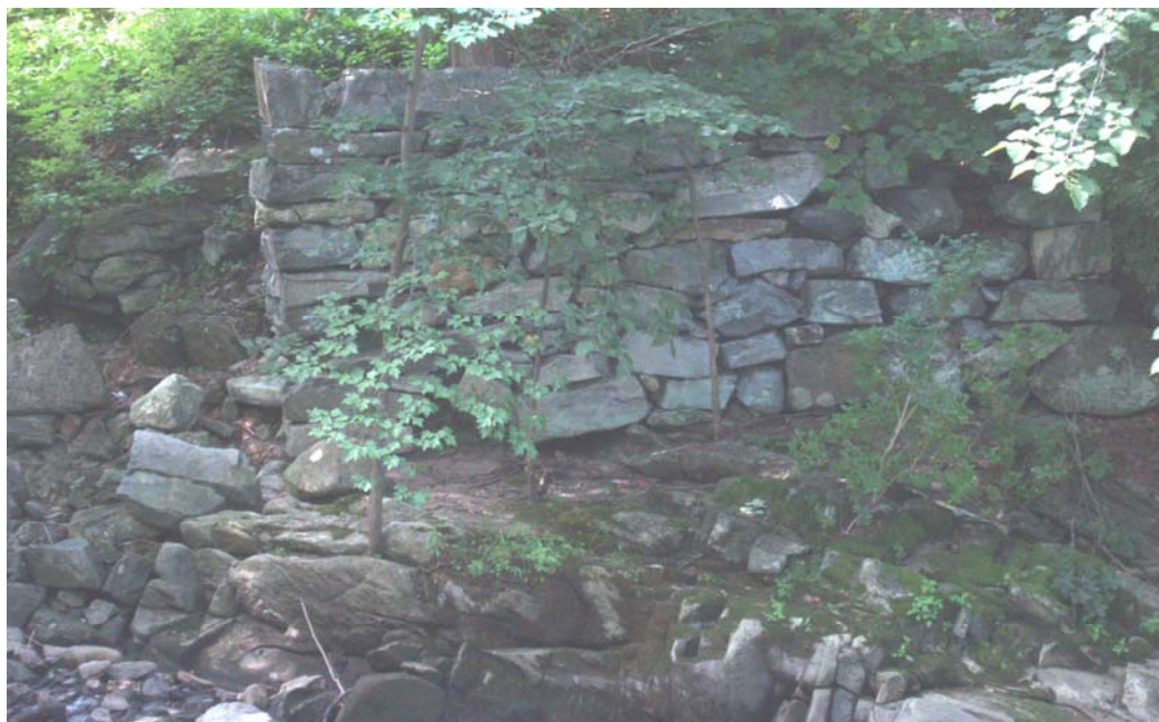
Figure No. 22: Southwest view of mill foundation on the steep west bank of the Still River in Brookfield village, constructed from roughly coursed stone.
