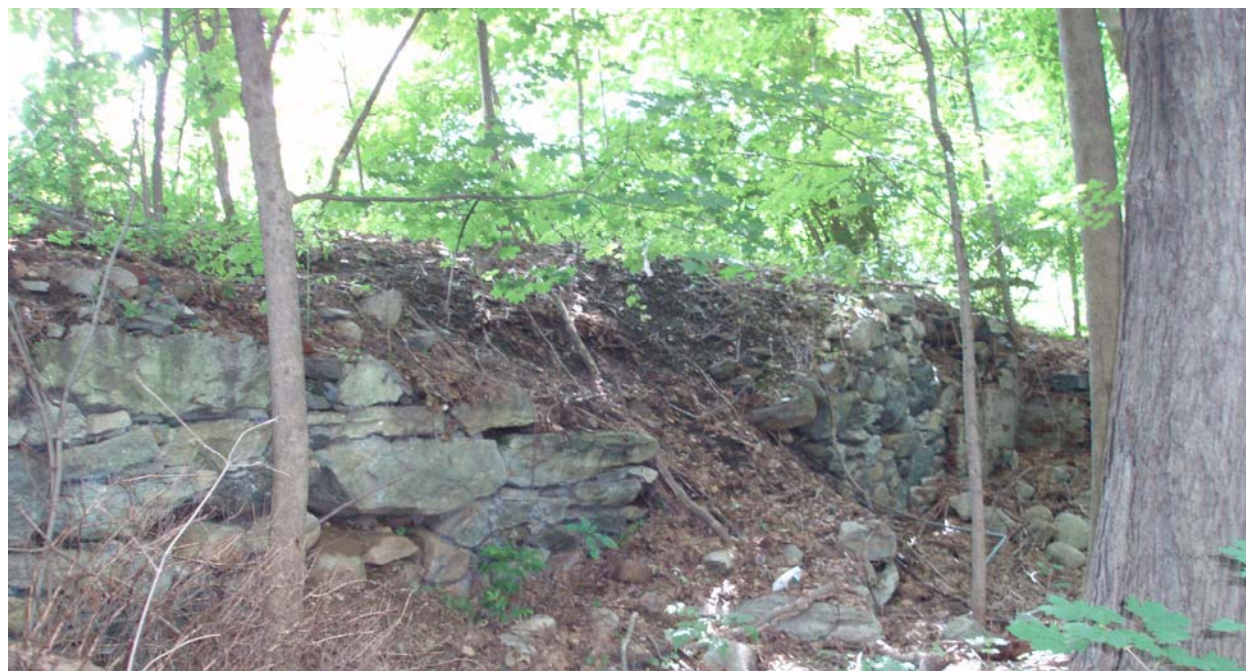
Figure No. 23: Southeast view of foundation NMF-1 in New Milford to the south of the town center. The southeast corner features an interior brick facing.
