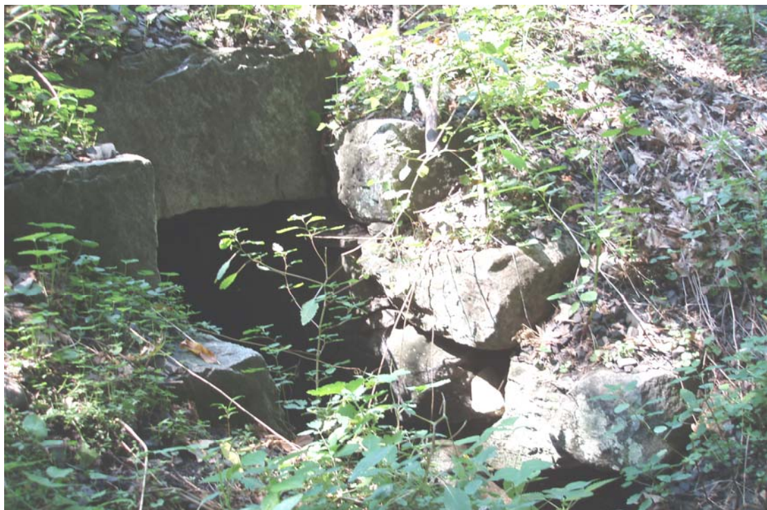
Figure No. 27: Northwest view of drainage culvert beneath railroad tracks, constructed from coursed stone. RR feature #47.
