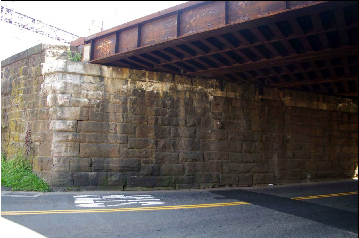
Figure 6. Fort Point Street Railroad Bridge, east abutment with ashlar stone masonry, camera facing southeast (AHS photograph, 9/2017).
