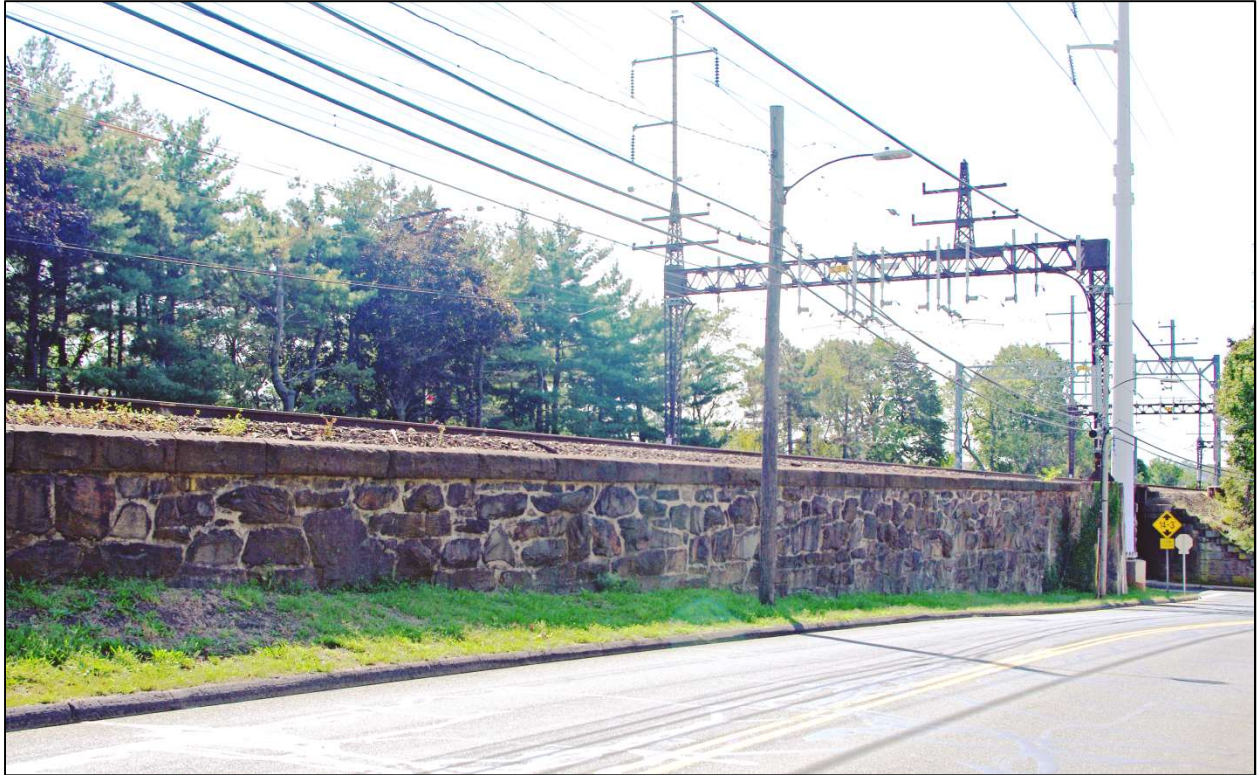
Photograph 4: Retaining wall east of Fort Point Street Railroad Bridge, camera facing southwest.
