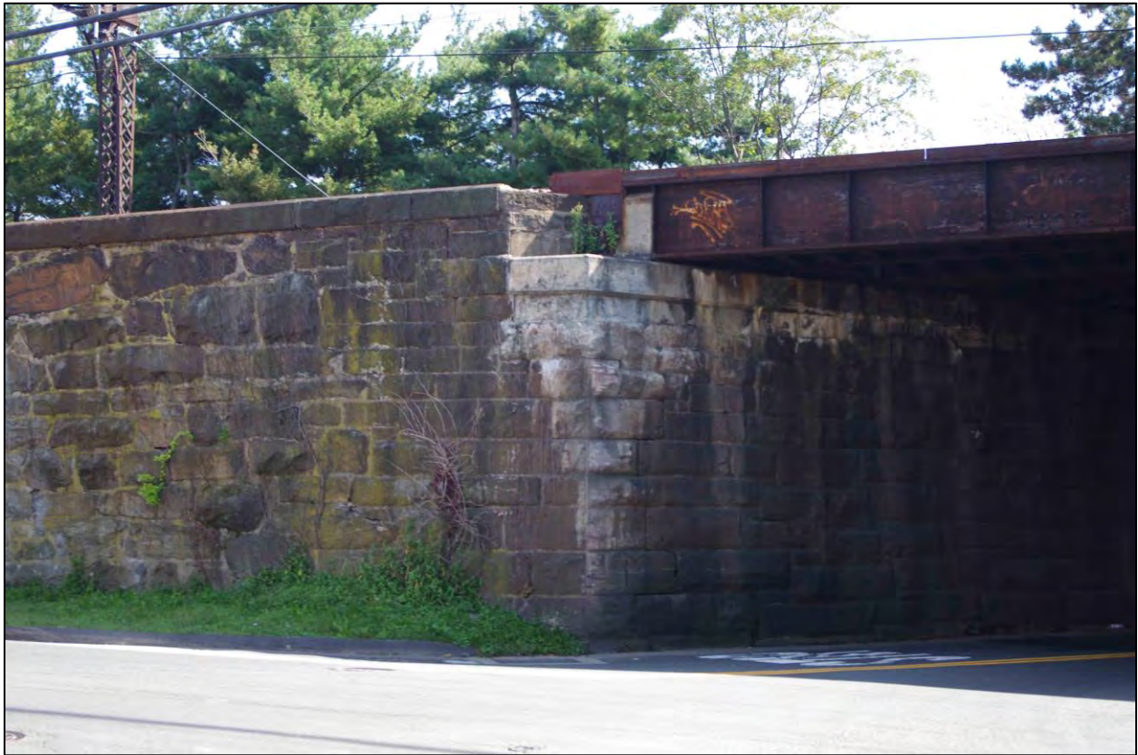
Figure 5. State-Level Documentation Photograph 24. Retaining wall east of Fort Point Street Railroad Bridge, detail of junction between the wall's rubble masonry and the bridge abutment's ashlar masonry, camera facing southeast (AHS photograph, 9/2017).
