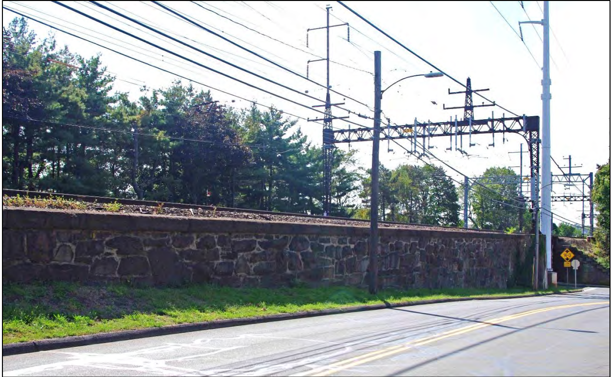
Figure 3. State-Level Documentation Photograph 22. Retaining wall east of Fort Point Street Railroad Bridge, camera facing southwest (AHS photograph, 9/2017).
