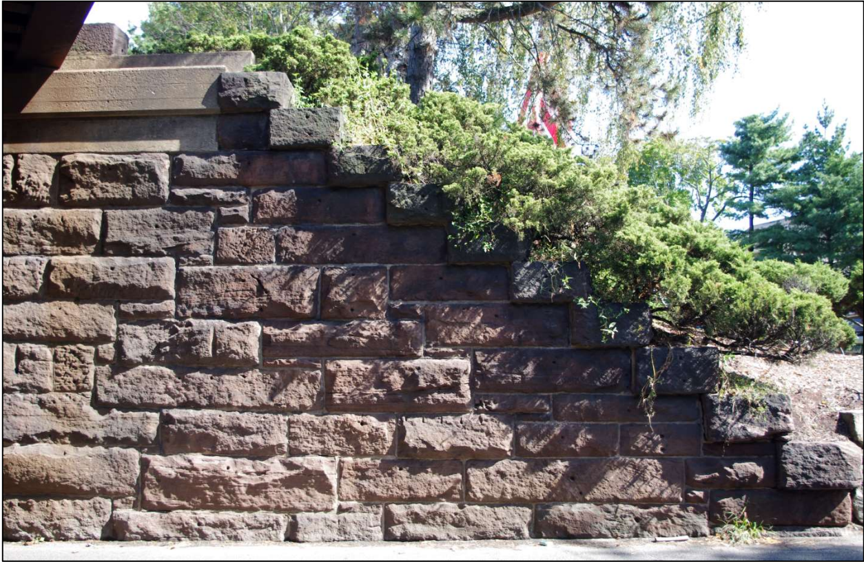
Photograph 2: Fort Point Street Railroad Bridge, detail of south end of east abutment, camera facing east.
