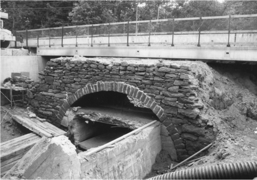
A concrete box culvert, here shown being removed, was inserted into the stone arch in the 1920s.
