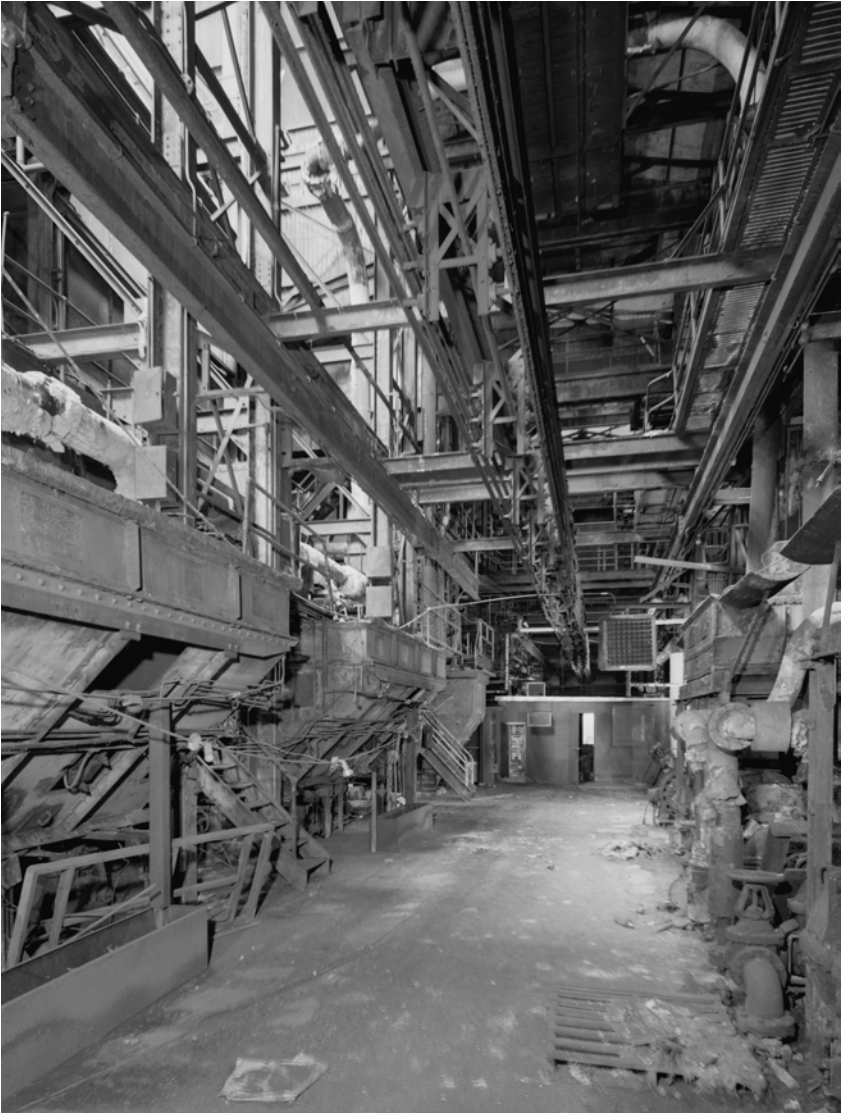
Firing aisle, east boiler room (HAER photograph by Jet Lowe).
