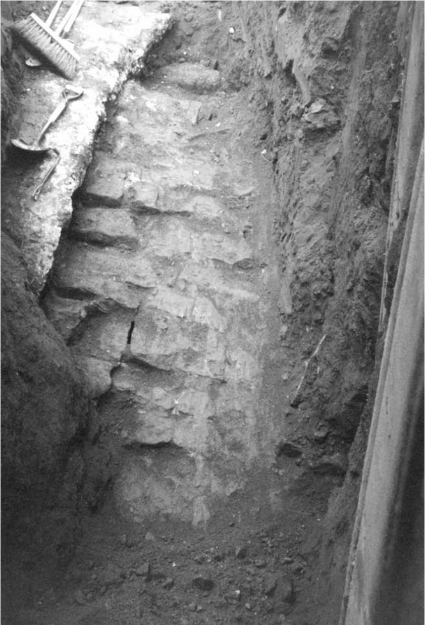
Exploratory excavation for the new bridge exposed sections of brownstone masonry just below the surface.
