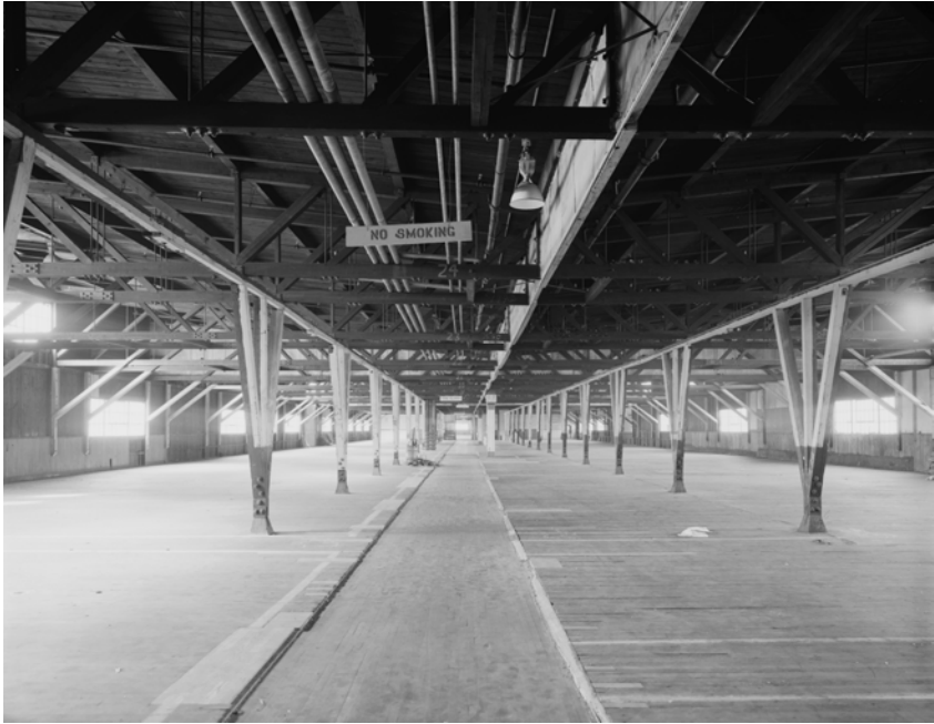
Interior, upper level, showing the warehouse's wooden framing (HAER photo by Robert Moore, 1993).
