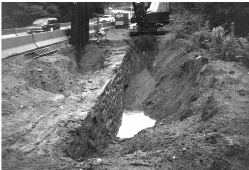
As fill was removed, more of the original stone arch came into view.
