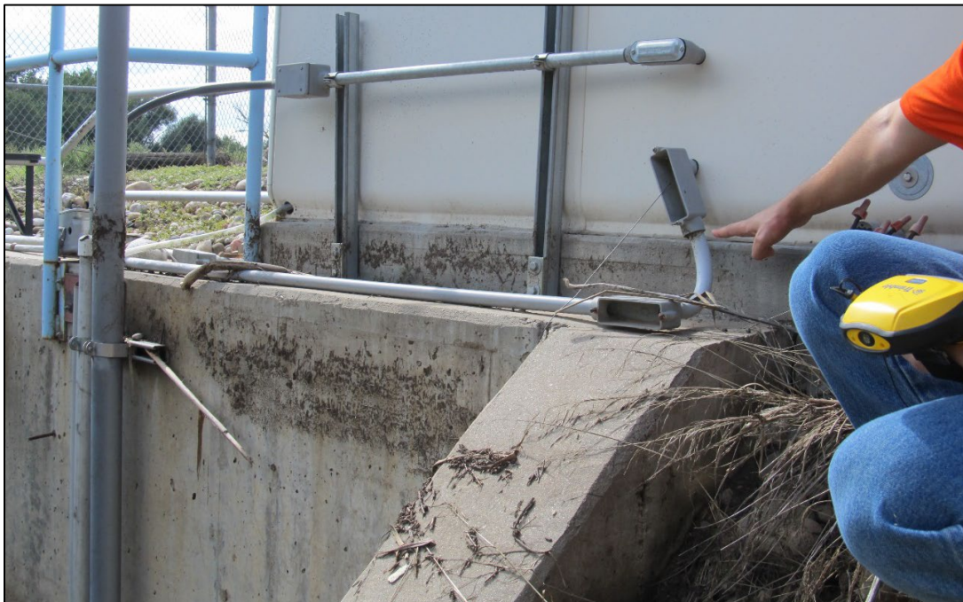
Figure 6.7. Mud line on building indicating high-water line.
