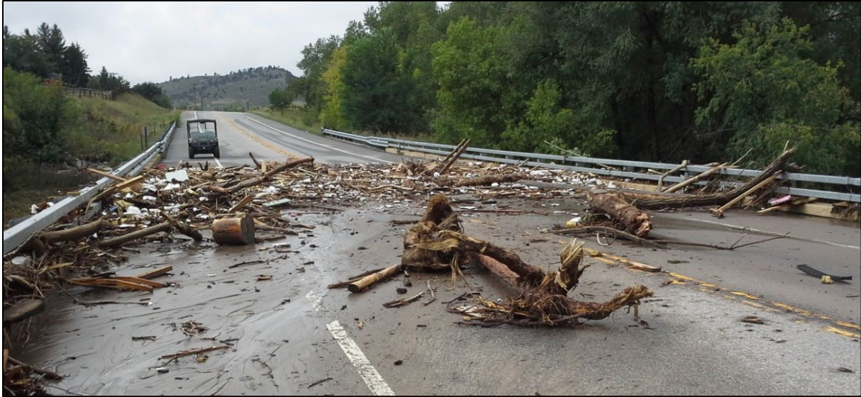
Figure 6.8. Flood debris on a bridge deck.
