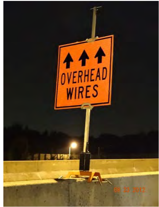
Median barrier clamping system for signs and safety sign used by contractor for trucks delivering materials. Good Practice
