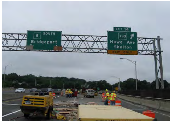
Figure 9: Minimal Protection from live traffic cluttered work area.
