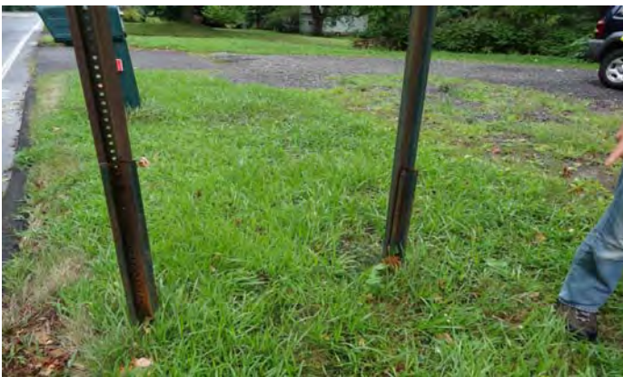
Height of breakaway posts is not according to plans.
