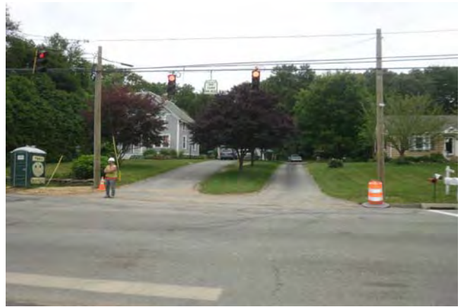
Temporary signalization for driveways
