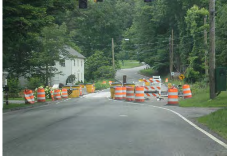
Type III Barricade with chevrons in wrong direction. Traffic Drum blocking DE-9.
