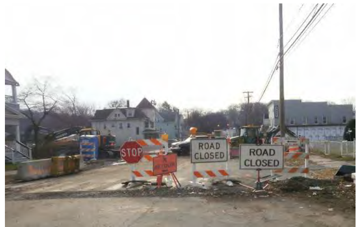
Sign No. 80-9929 to inform the public of the bridge closure. In accordance with Note 9 on the plans, this sign should have been removed once the detour was in effect.
