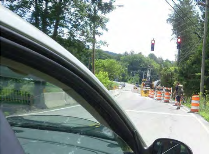
Notice Blunt end on Temporary Precast Concrete Barrier Curb.
