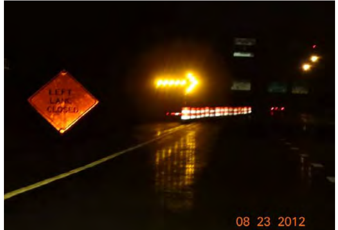
Sign too close to lane closure.
