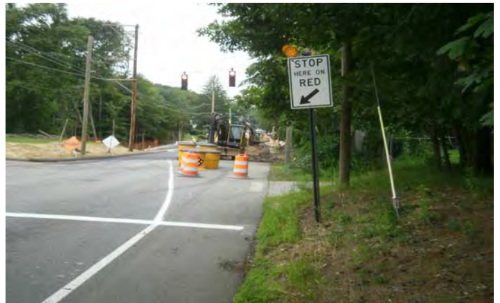
Proper placement of sign and pavement markings for temporary signalization at bridge Notified inspector about traffic barrel blocking view of Delineator
