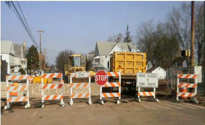
Type III barricades and signs placed at south end of bridge. Barricade stripes should all be sloping downward in the direction traffic is to pass (in this case to the left) and be retroreflective.
