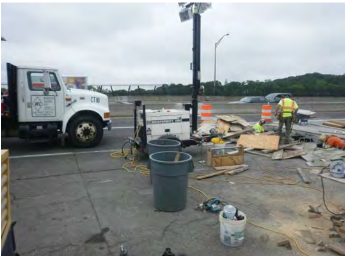
Figure 7: Cluttered Work Area
