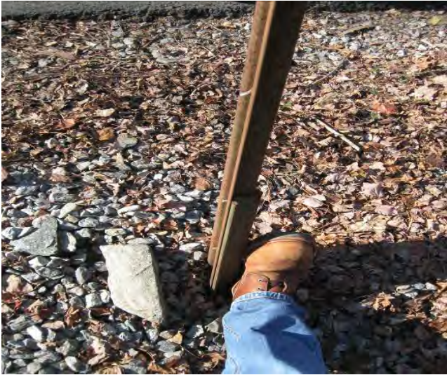
Improper breakaway post height.
