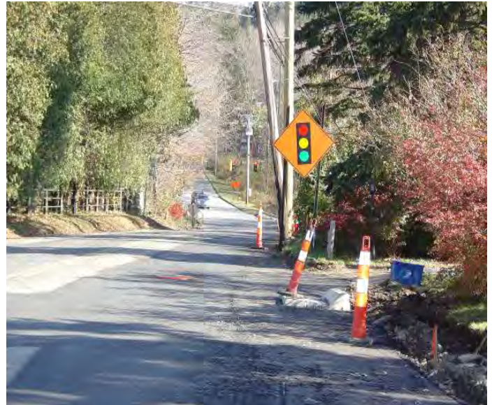
Utility Pole leaning; town road used for detour.
