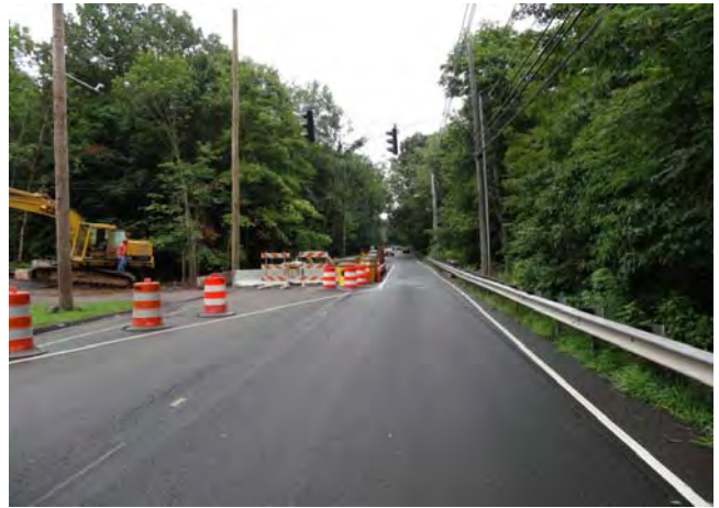
DE-9 delineator is temporarily blocked by the barrel. Type III barricade on the right has striped pattern sloping in the opposite direction.
