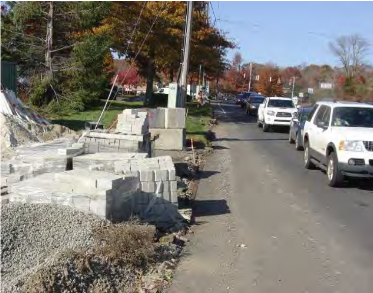
Material too close to Roadway
