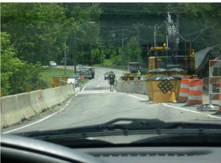
Hiker Access to Kent from the Appalachian Trail, Design did not consider this.
