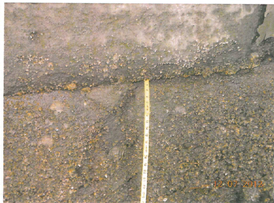
Photo No. 14: Typical Missing Mortar in Stone Masonry
