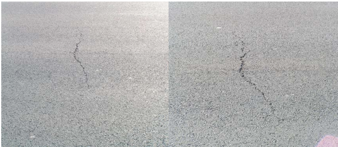
Winter '08 & '09 Transverse Crack
