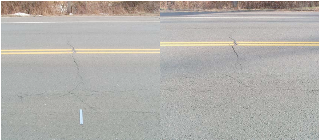
Winter '08 &'09 Transverse Crack
