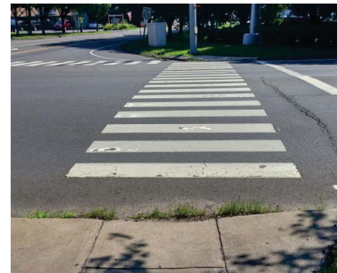
Figure 7. Ramp Missing Detectable Warning Strips/no Sidewalk Connection at Ramp Landing
