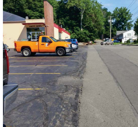
Figure 5. No Driveway Curb Cut
