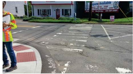
Figure 11. Worn Crosswalk Paint/ crosswalk Does Not Lead to Ramp Landing (northeast corner)
