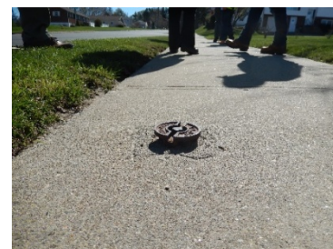
Figure 8: Utility access point obstruction
