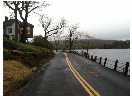
Figure 13. Tight corner, failing cable guard rail
