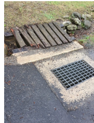
Figure 9. Unusual drainage structures
