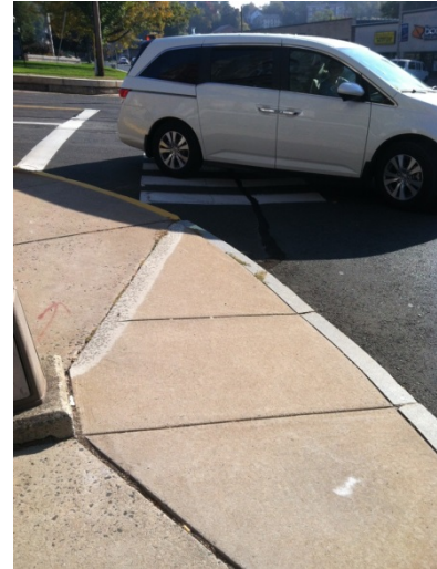
Figure 5. Crosswalk not Meeting Ramp on the Northwest Corner of the West Main Street, Elm Street and Union Street Intersection
