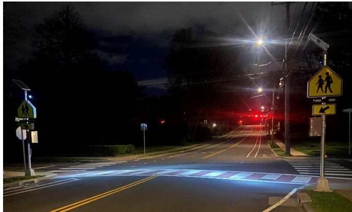
Exhibit 24: An example of a crosswalk high intensity light integrated with an RRFB at night in West Hartford, CT. Note – The yellow flashers are not activated in this photo to demonstrate the crosswalk light.
