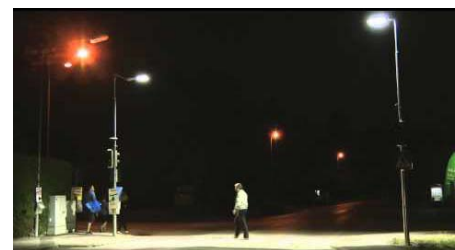
Figure 31. LED Lighting at Crosswalk
