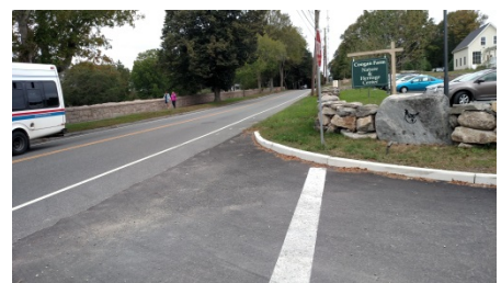
Figure 30. Inadequate Sight Distance for Potential Crosswalk
