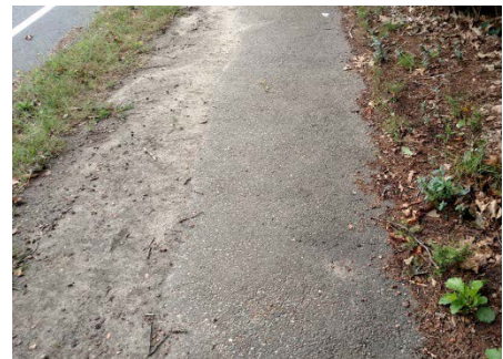
Figure 10. Clearing and Grubbing Needed on Sidewalk
