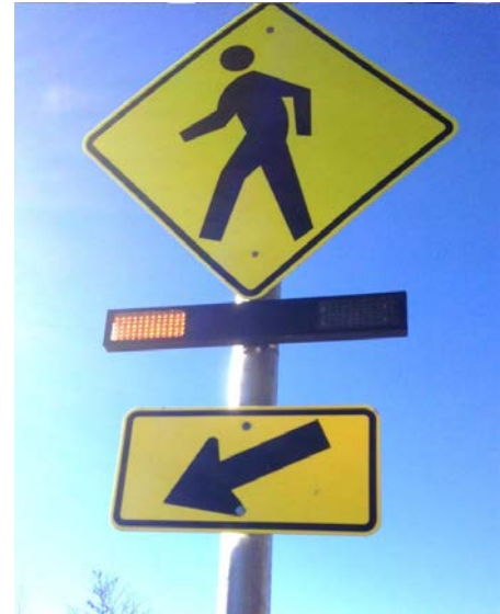
Figure 38. Active Pedestrian Crossing Sign
