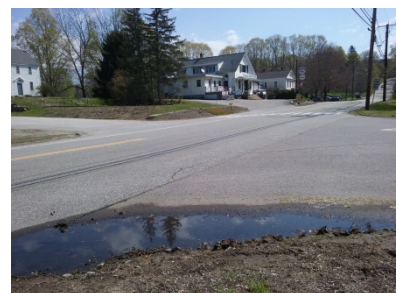
Figure 10. Drainage Issues at Center Street and Route 14
