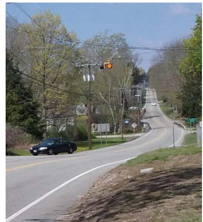
Figure 9. Flashing Beacon at Route 97 & 14
