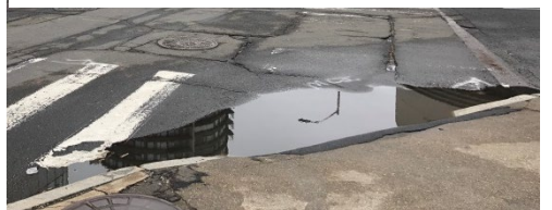
Figure 14: Detectable warning strip missing and poor drainage
