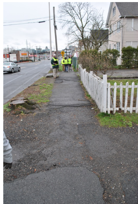
Figure 11: Poor sidewalk condition
