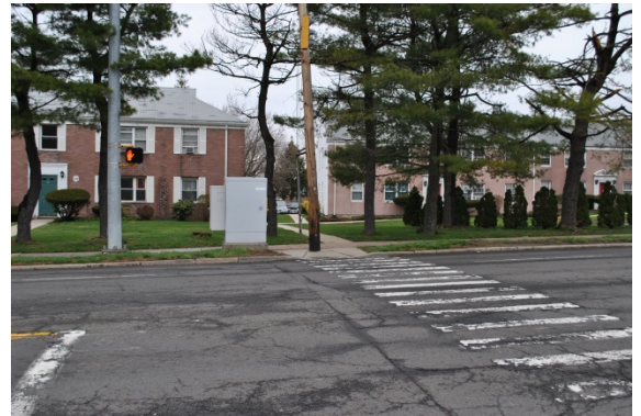
Figure 8: Utility poll blocking pedestrian sidewalk ramp
