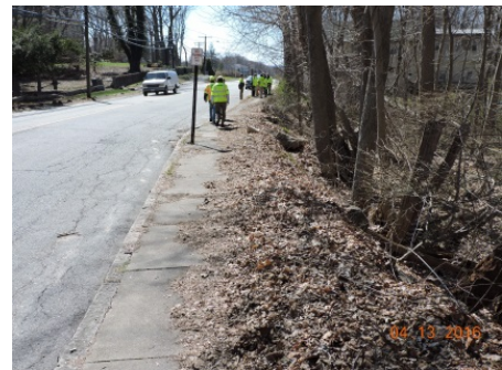
Figure 22. Steep Drop-off Adjacent to Sidewalk
