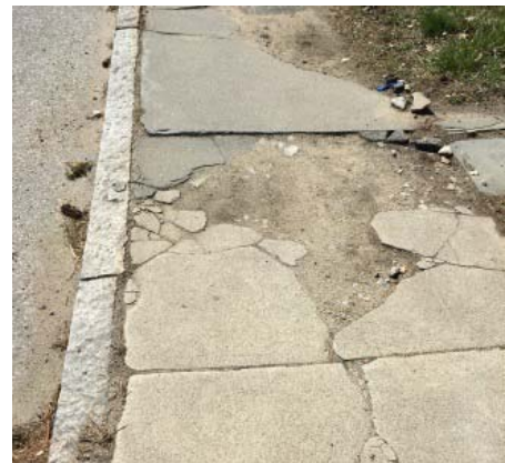
Figure 19. Poor Sidewalk Conditions Along Williams Street
