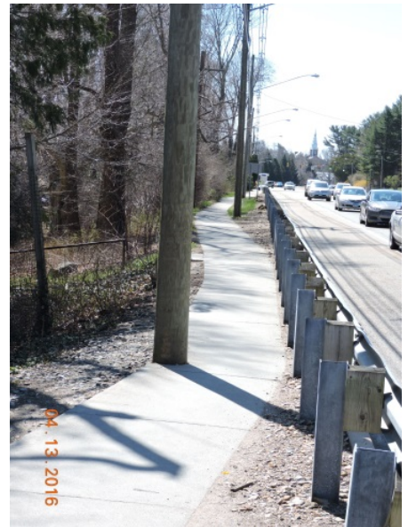
Figure 10. Utility Poles in the Sidewalk Path
