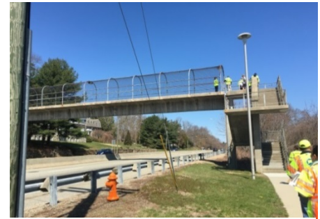
Figure 8. Pedestrian Bridge, not ADA Compliant
