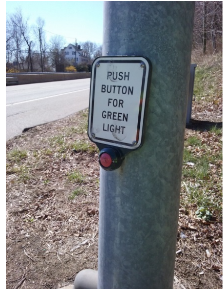
Figure 6. Pedestrian Push Button for Crossing
