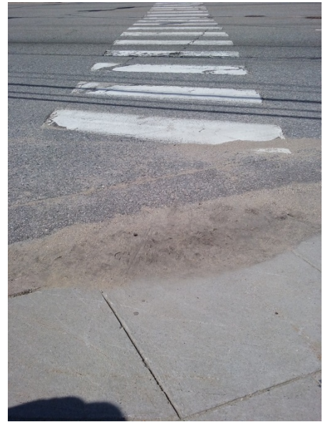
Figure 29. Non-ADA Compliant Crosswalk
