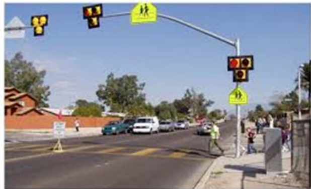
Figure 49. Example of Hawk Crossing System
