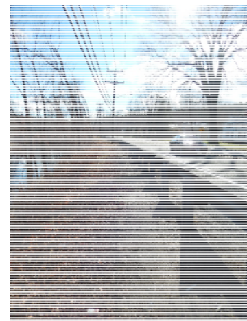
Figure 20: Route 44 looking south of Upcountry Sports Fishing Store on the east side
