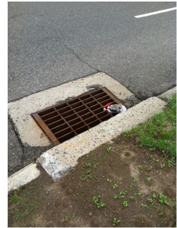
Figure 7. Non-bike friendly catch basin grate
