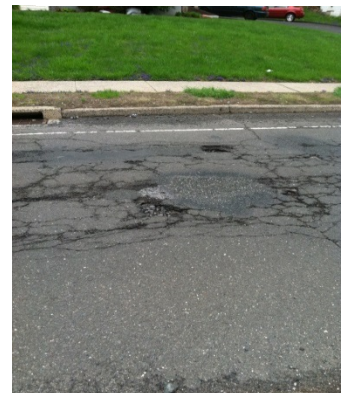
Figure 12. Poor pavement condition
