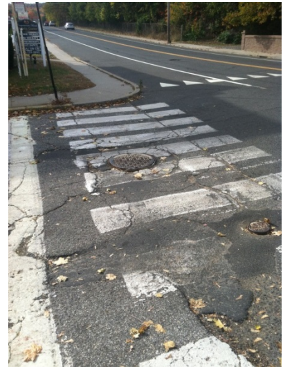
Figure 10. Crosswalk without ADA compliant ramp or warning strips
