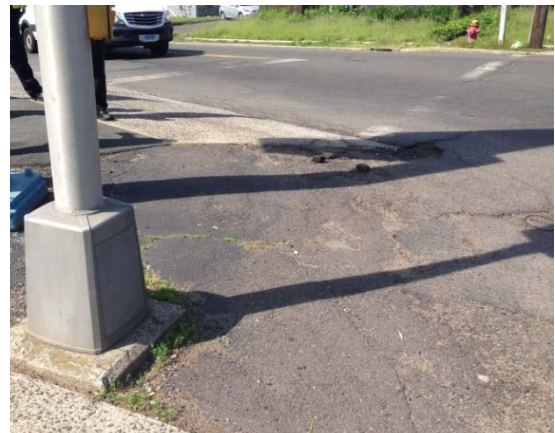
Figure 10. No sidewalk ramps
