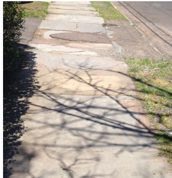
Figure 11. Sidewalk in poor condition
