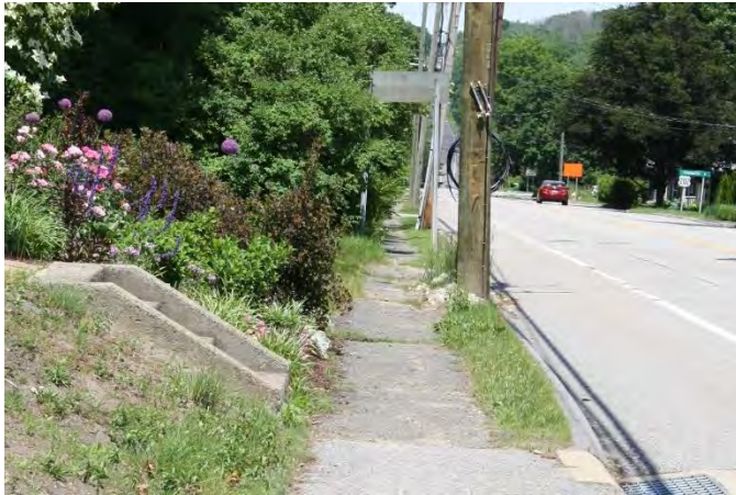
Figure 25: Sidewalk conditions on Torrington Road (Route 202) north of East Street (Route 118)
