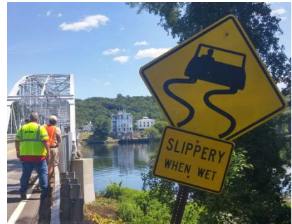
Figure 18. Drop off on South Side of Swing Bridge (West End)
