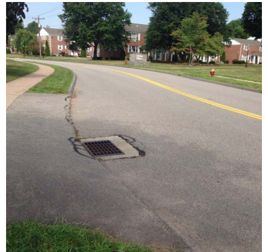
Figure 10: Catch Basin in the Driveway
