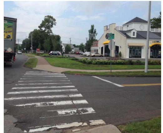
Figure 6: Deteriorating Pavement Markings
