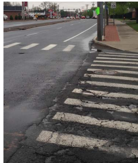
Figure 9. Poor Pavement and Crosswalk Conditions at Willis Street
