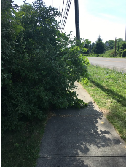
Figure 17. Trim areas with overgrown vegetation
