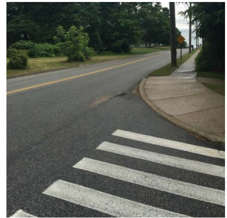
Figure 13. Lack of Detectable Warning Strips
