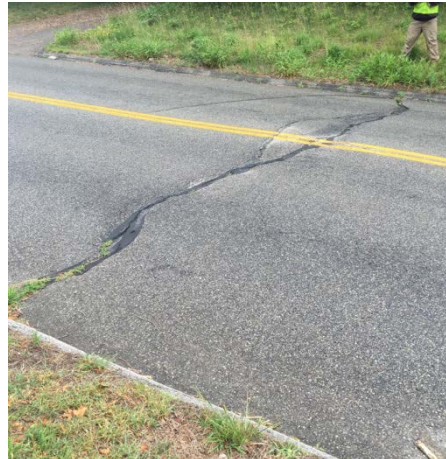
Figure 17. Horizontal Crack in Road
