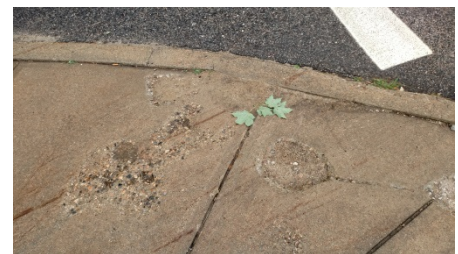
Figure 15. Broken Sidewalk Ramp
