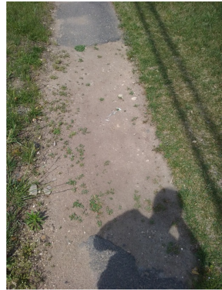
Figure 16. Sidewalk Along Dowd Avenue in Poor Condition
