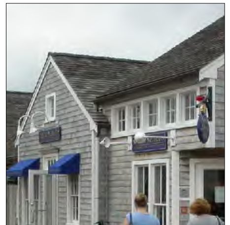
Wall sign lighting
