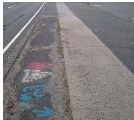
Figure 12. Sidewalk Along Route 44 Which Provides an Unwelcoming Feeling
