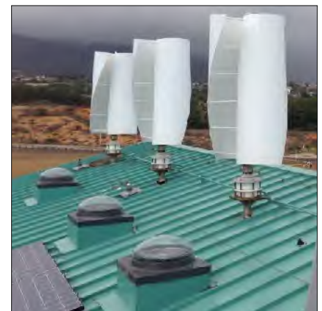
Rooftop wind turbines
