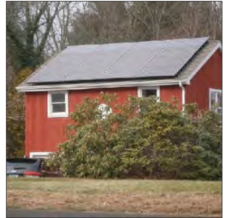
Photo-voltaic (solar) panels
