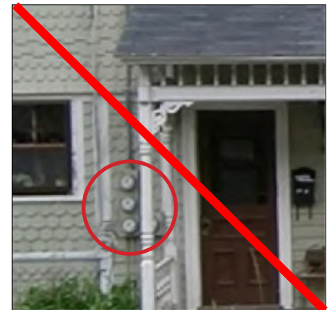
No electrical equipment on front facade
