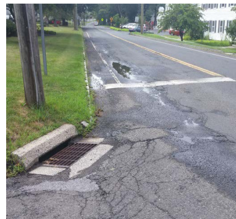
Figure 15. Drainage issues and pavement rutting on northbound Route 133 approach to Clapboard Road.
