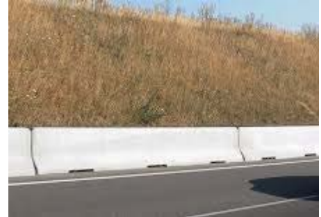
Figure 24: Safety Shape Barrier
