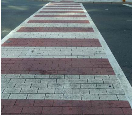
Figure 22. Example of Painted and Textured Crosswalk
