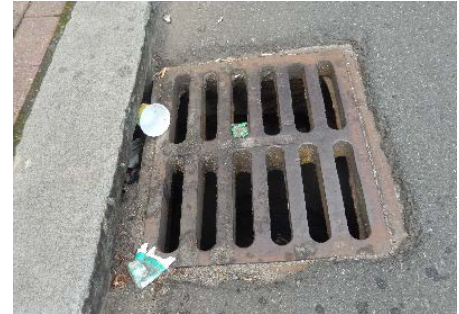
Figure 20. Non-Bike Friendly Catch Basin Grate
