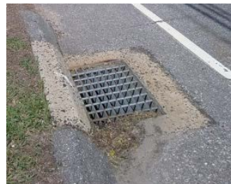
Figure 29: Bike friendly catch basin
