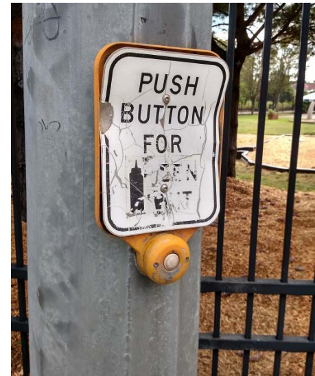
Figure 9. Broken Pedestrian Push Button
