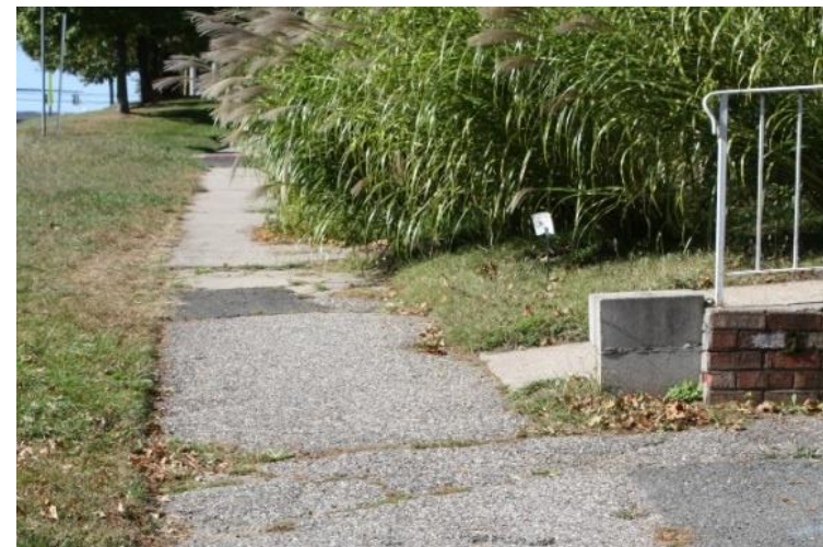
Exhibit 21: Sidewalk in poor condition on the north side of Route 1
