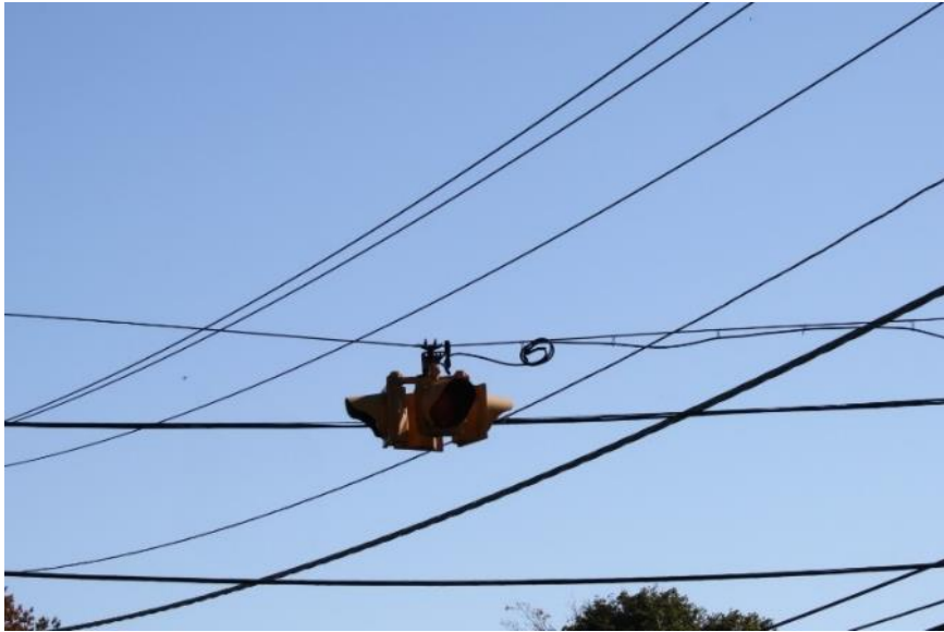
Exhibit 23: Inoperable flashing beacon at Ridgefield Avenue
