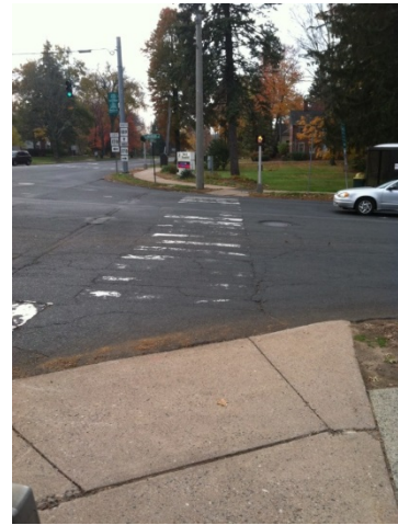
Figure 8. Faded crosswalk at intersection
