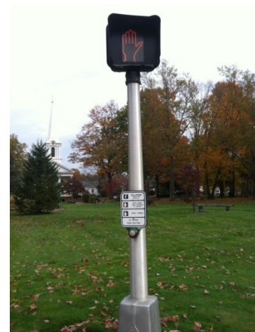
Figure 7. Pedestrian pushbutton and signal
