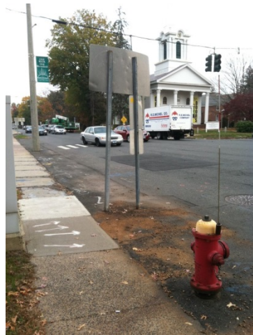
Figure 9. Diagonal crosswalk at intersection; poor sidewalk condition
