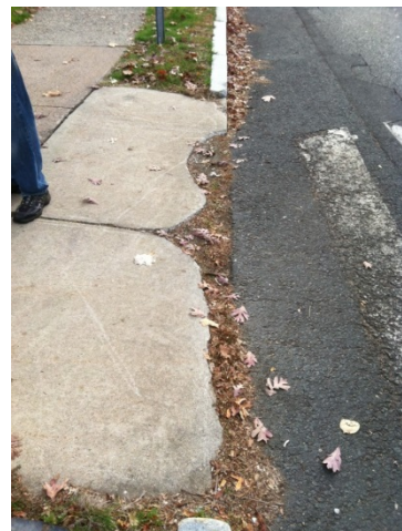
Figure 10. Damaged handicap ramp, no detectable warning strips
