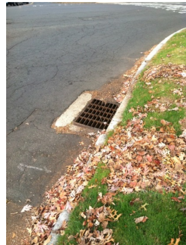
Figure 6. Catch basin grate at intersection
