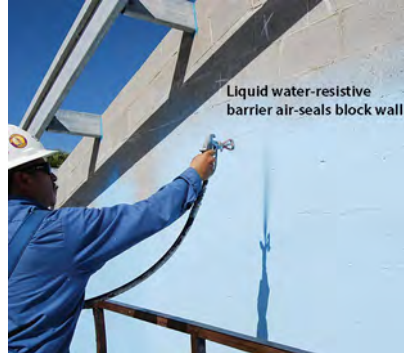
Liquid water-resistant barrier: This retrofit serves two purposes: water proofing and air sealing.
