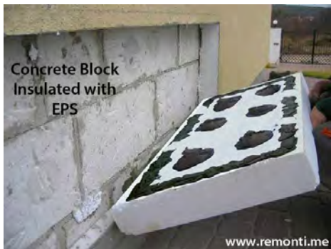
EPS foundation insulation: Installers glue masonry-faced EPS-foam sheets to the block wall.
