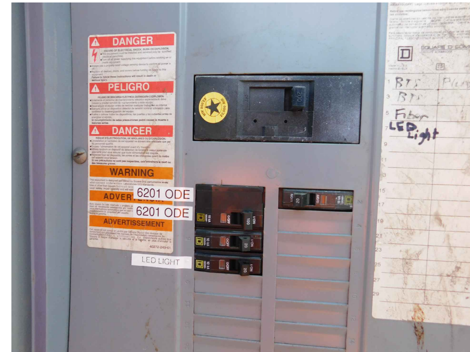
EXISTING POWER PANEL PHOTO
