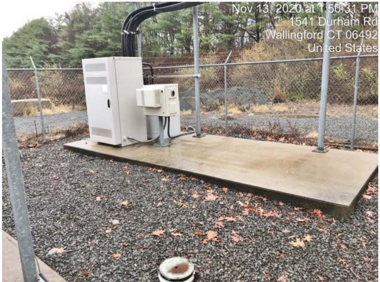
Existing T-Mobile Equipment Cabinets Mounted To Existing Concrete Pad
