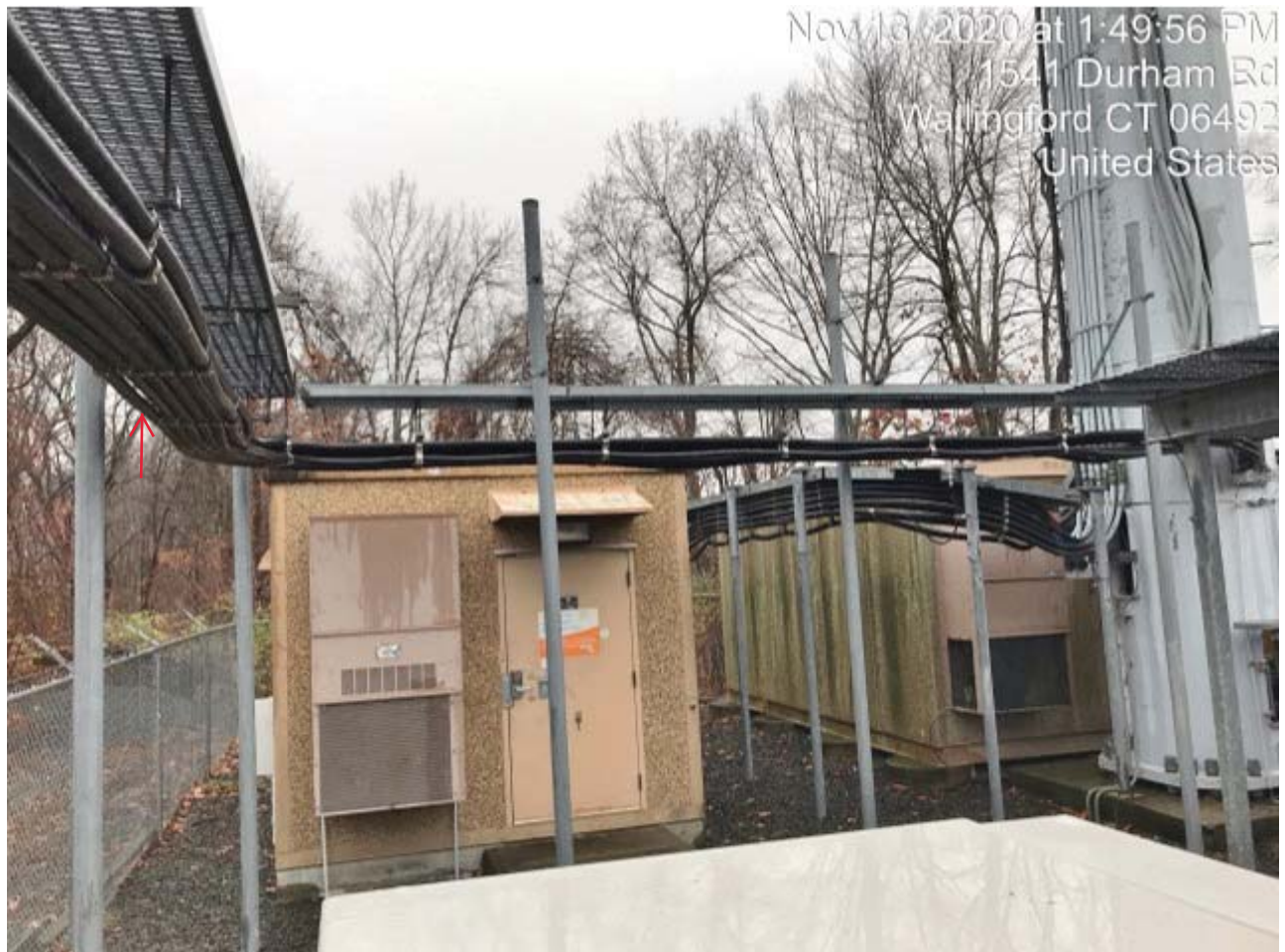
(1) New Signal Cable Routed Along Existing Ice Bridge From The Cabinet To The Monopole
