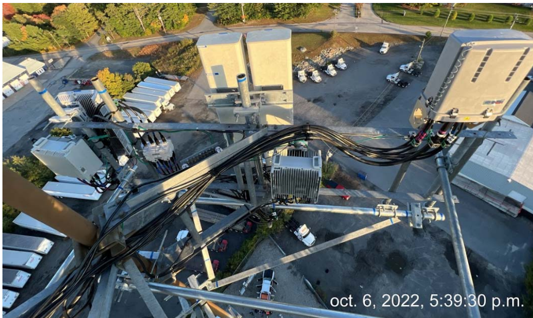
Fig. 2: Overall View of Antennas, RRHs & OVP in Beta Sector
