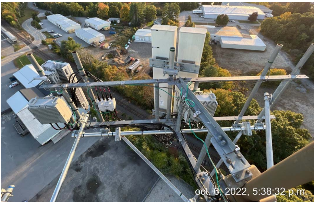
Fig. 3: Overall View of Antennas, RRHs & OVP in Gamma Sector
