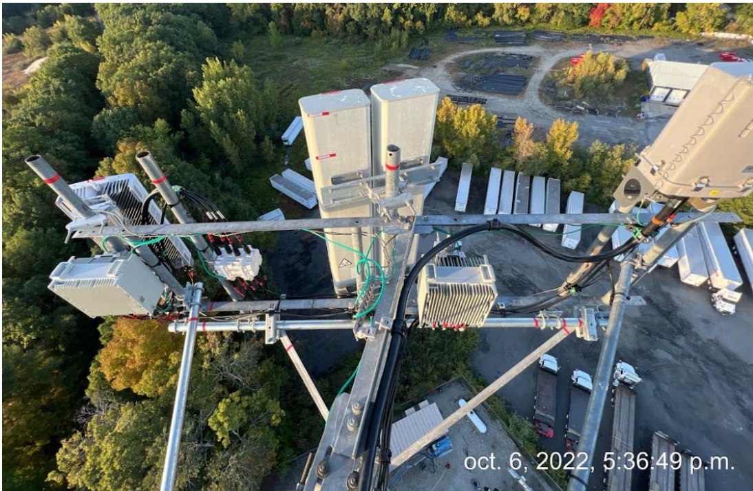
Fig. 1: Overall View of Antennas, RRHs & OVP in Alpha Sector
