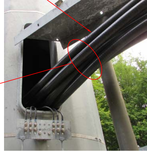
FEEDLINE PHOTO DETAIL AT TOWER BASE SCALE: N.T.S. 3 A-1
