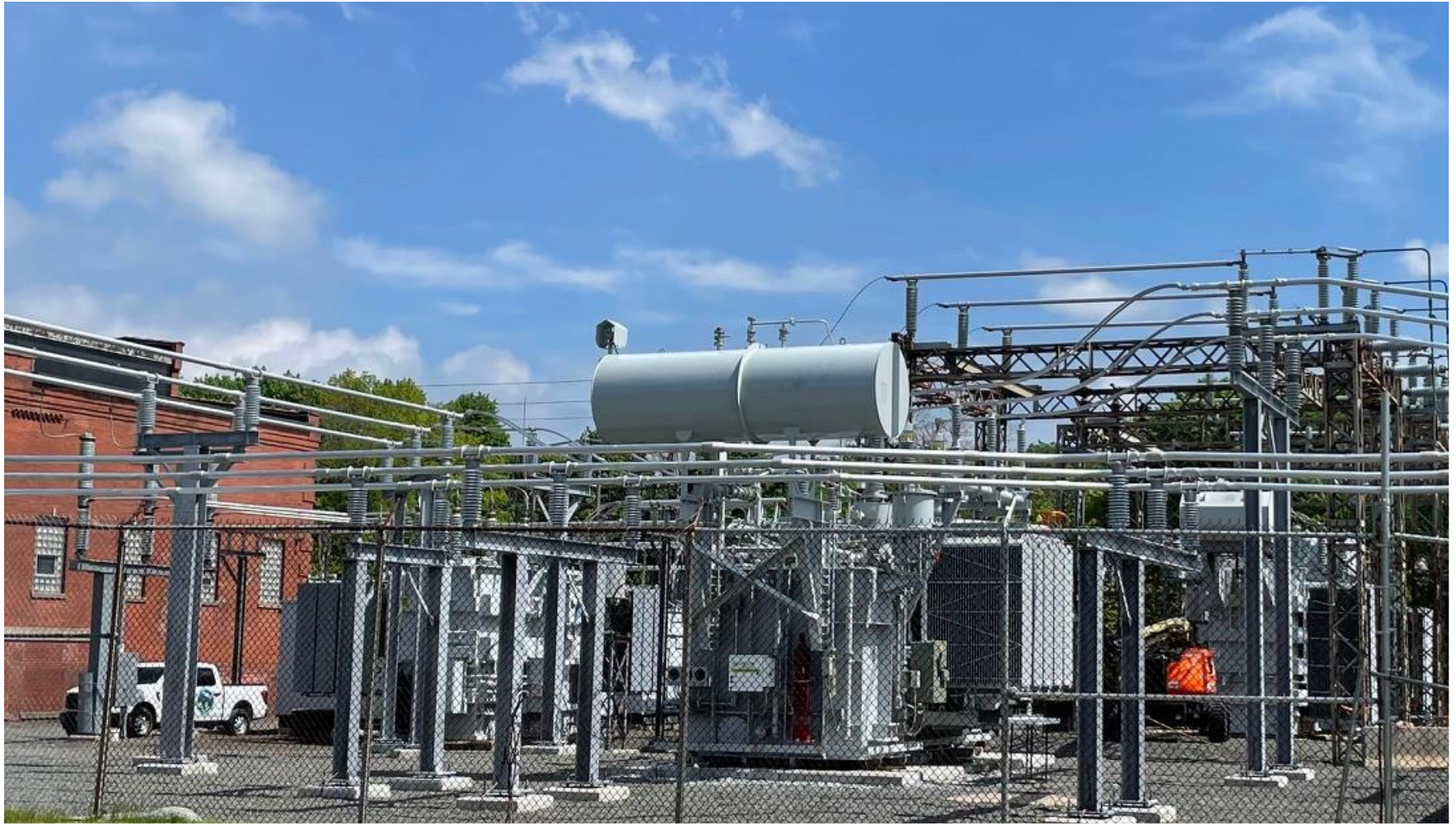
Attachment A: Photograph of Replacement Transformer: Black Rock Substation
