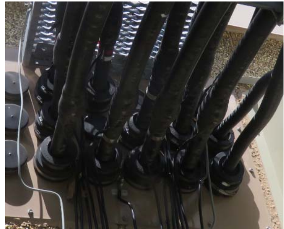
Verizon Cable entry at shelter
