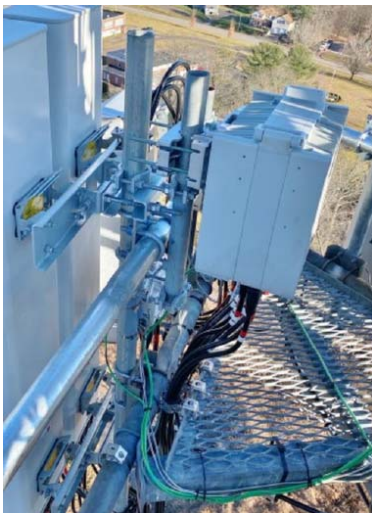
RRH mounted to separate pipe which differs from original design, but is an acceptable installation.
