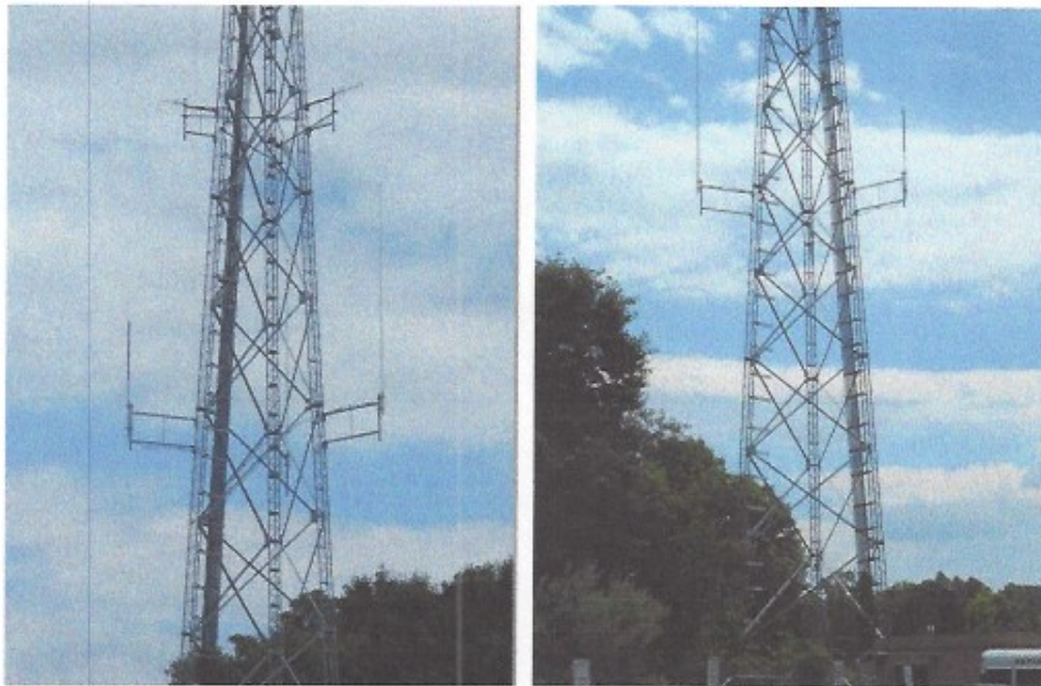
Photos showing equipment on lower tower.
