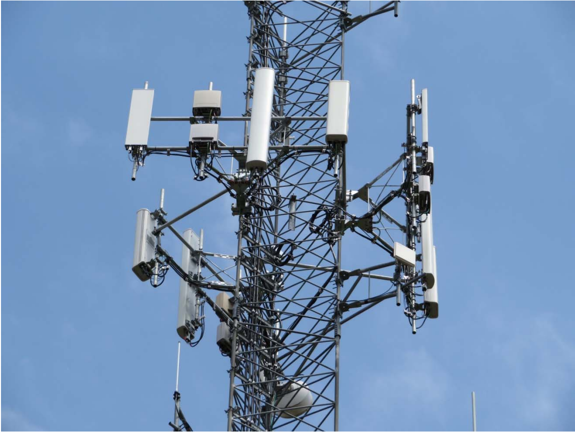
Photo 1: Photo illustrating the Tower with Appurtenances shown.
