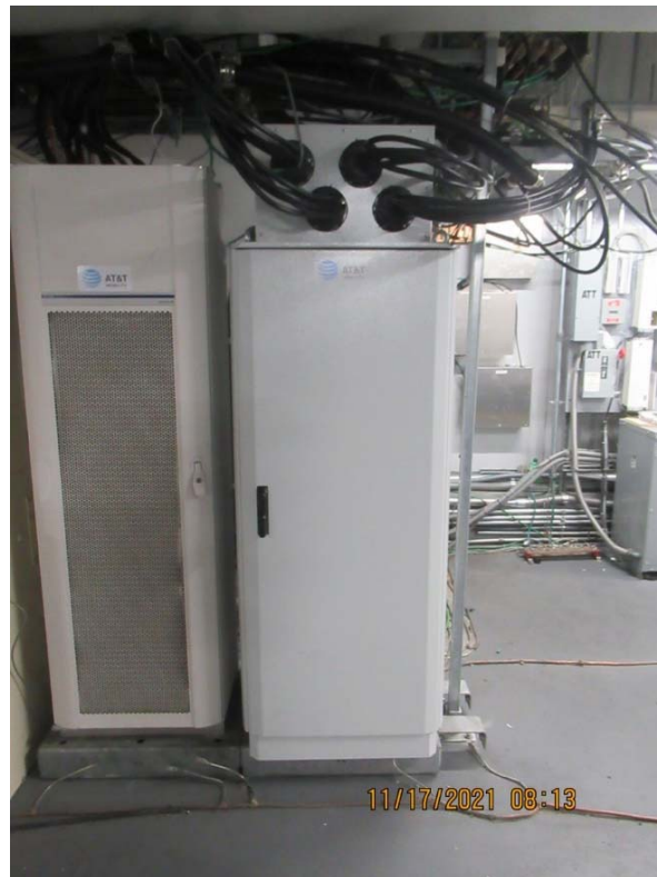
Photo 4: Sample photo illustrating the existing equipment cabinets.
